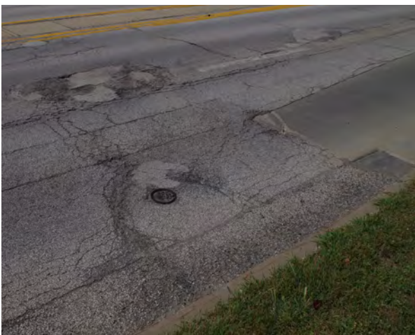
Left: The pavement along Fairway Drive is deteriorated.
