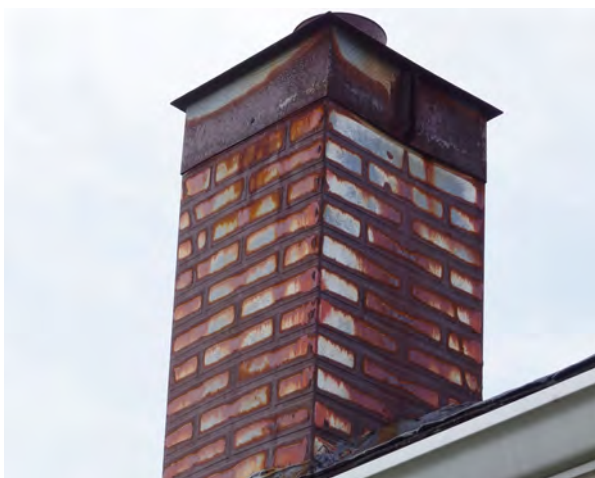
Left: The chimney cap on the Moose Lodge has rusted and stained the entire chimney. (614 IAA Drive)
