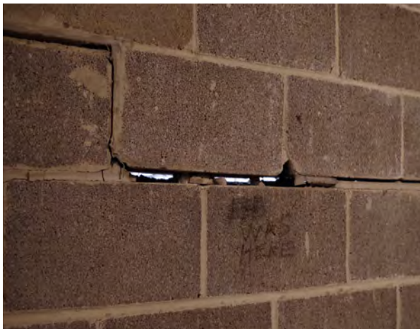
Left: A crack in the concrete block wall allowing light to pass through K-Mart. (1608 East Empire Street)
