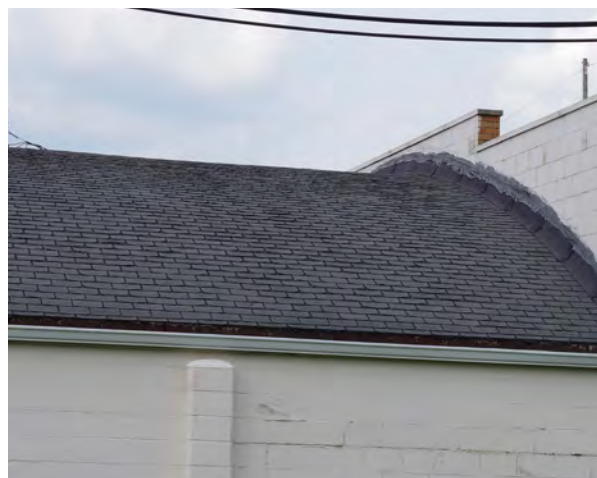
Right: The shingles on the roof of the Moose Lodge are deteriorated. (614 IAA Drive)
