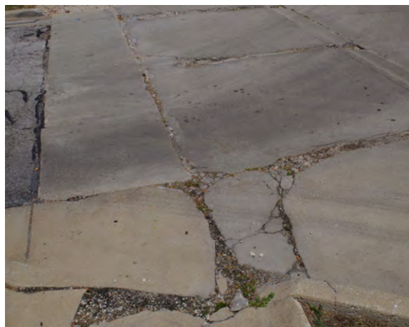
Right: The apron leading from IAA Drive to the eastern entrance Colonial Plaza is severely deteriorated.
