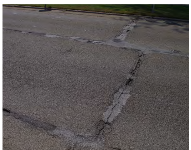
Right: Deteriorated pavement at the intersection of Empire and Towanda.
