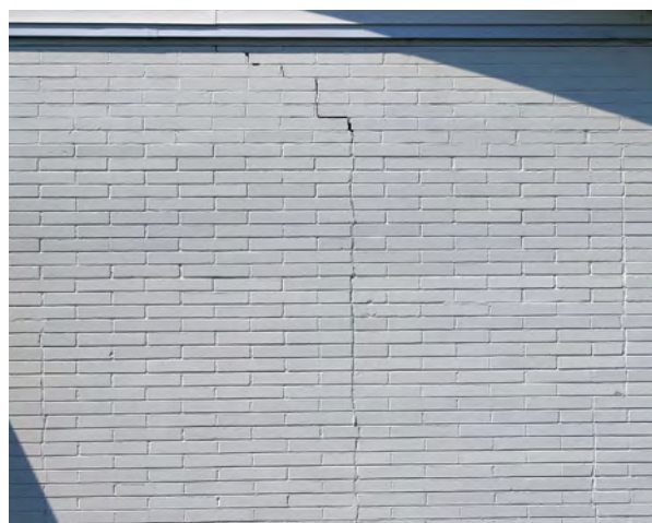
Right: Cracking in the exterior brick wall of this multi-tenant building. (1328 East Empire Street)
