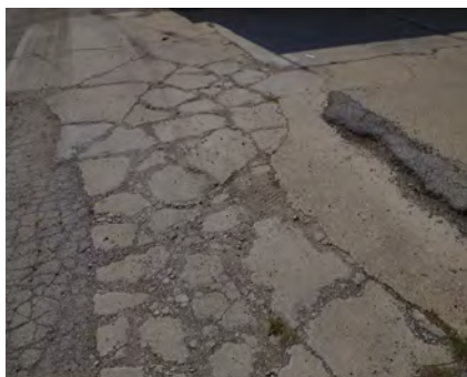
Below: The rear parking area at the post office is deteriorated. (1212 Towanda Avenue)
