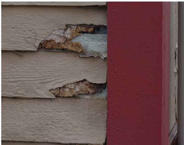
Left: The siding on Bandana's BBQ is deteriorated. (502 IAA Drive)
