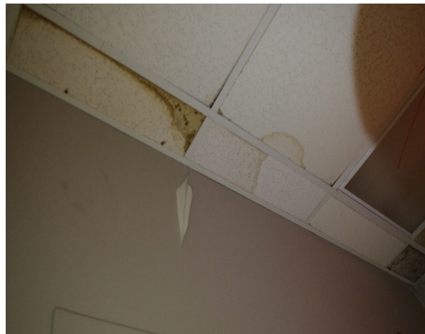
Right: Water damage to the interior ceiling tiles of the former Circuit City. (1500 East Empire Street, Suite 1A)
