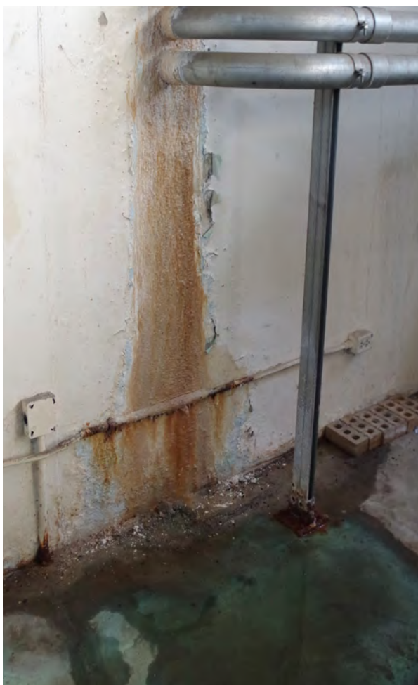
Left: Water seeping through the foundation wall of the boiler room at Bloomington High School. (1200 East Locust Street)
