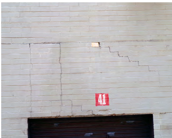
Left: Step cracking in the rear of the former K-Mart. (1608 East Empire Street)
