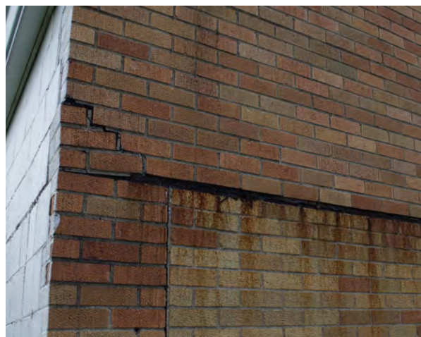
Right: Cracking in the exterior brick wall of the Moose Lodge. (614 IAA Drive)
