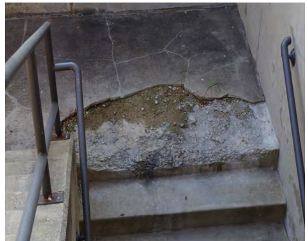
Right: The concrete of this stairwell at Bloomington High School is disintegrating.
