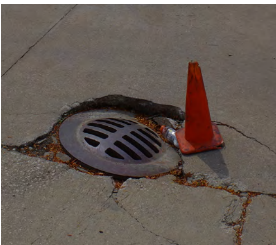
Left: The pavement around this storm drain at the Baymont Inn is broken and inlet cover is sinking. (604 IAA Drive)
