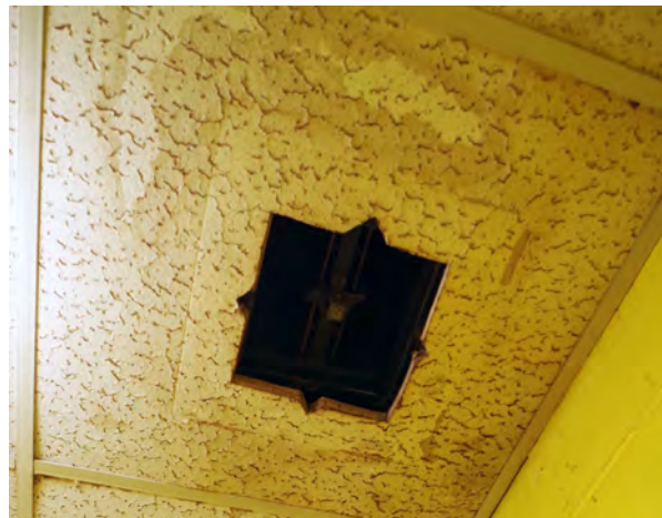
Right: Water damage to the interior ceiling tiles. (1500 East Empire Street)
