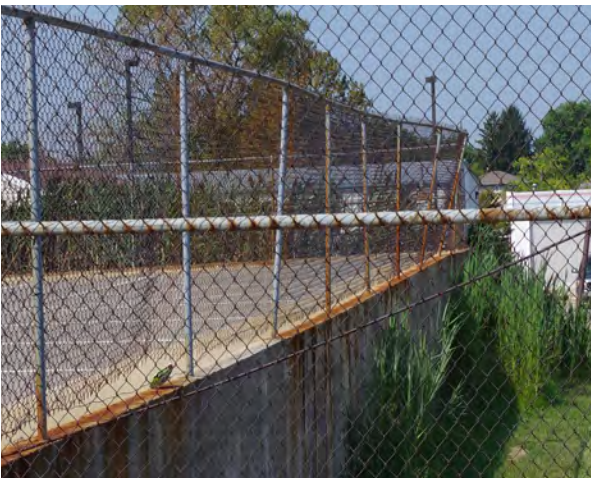
Left: The fence surrounding the post office distribution center is deteriorated. (1511 East Empire Street)
