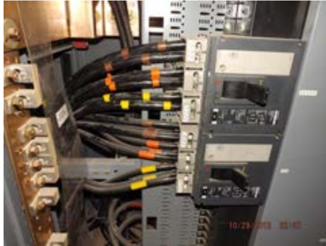
Figure C-2: Ice Plant Breaker
