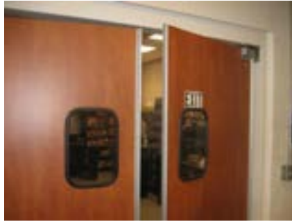
Figure-10 : Main Kitchen Doors Held Open by Air Pressure Imbalance
