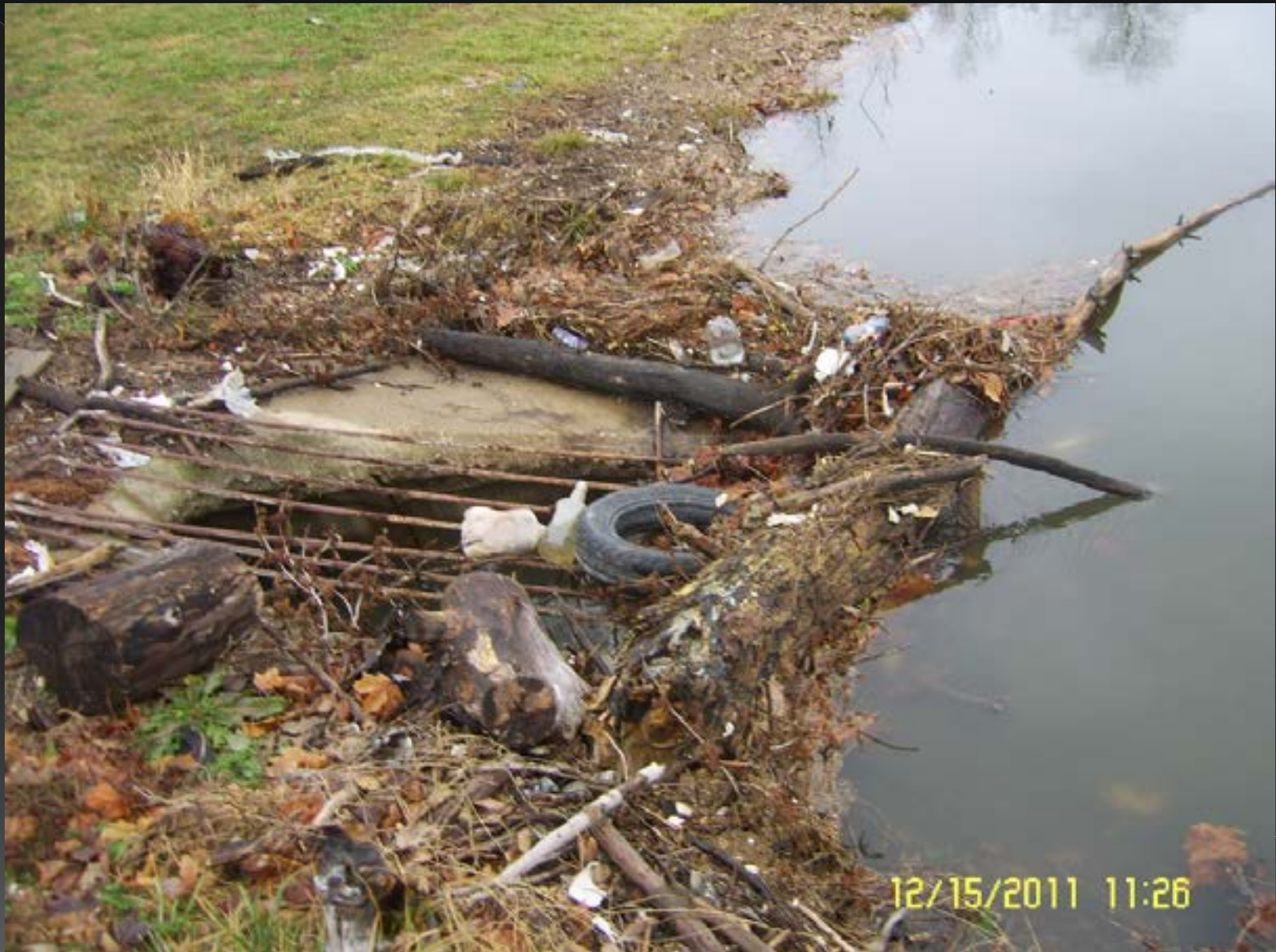
Baker-Ash detention basin. Without proper maintenance, washed-up debris inhibits drainage.
