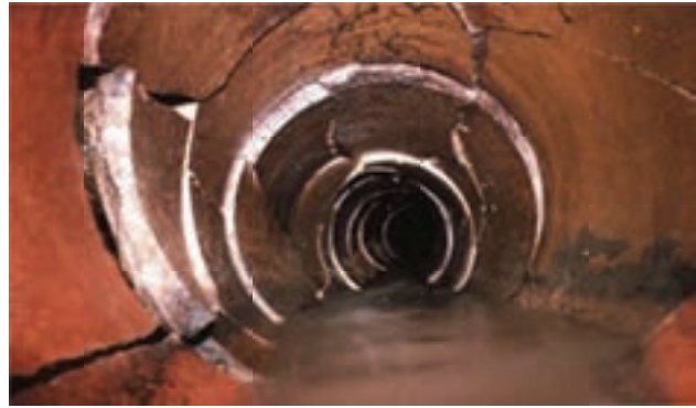
Figure 1 Deteriorated Sanitary Sewer Pipe
