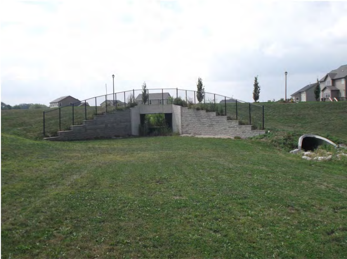
Grove 2 nd Addition - Pedestrian Underpass and Drainage Culvert below Black Oak Boulevard
