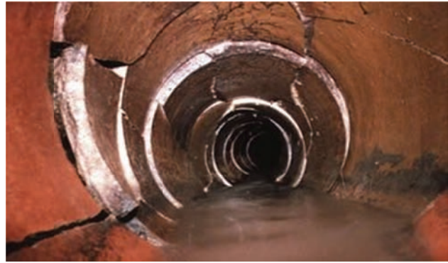
Figure 1 Deteriorated Sanitary Sewer Pipe
