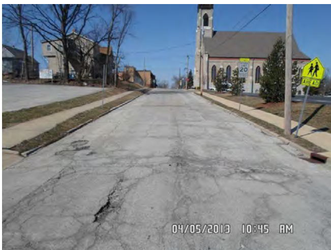
Figure 8 - Jackson Street prior to CRF treatment
