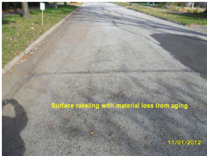
Figure 6 - Moore Street prior to 70/30 CRF treatment
