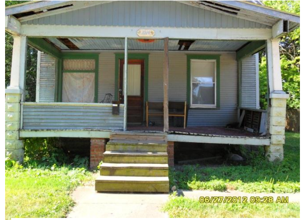
Deteriorated and Unsafe Front Porch
