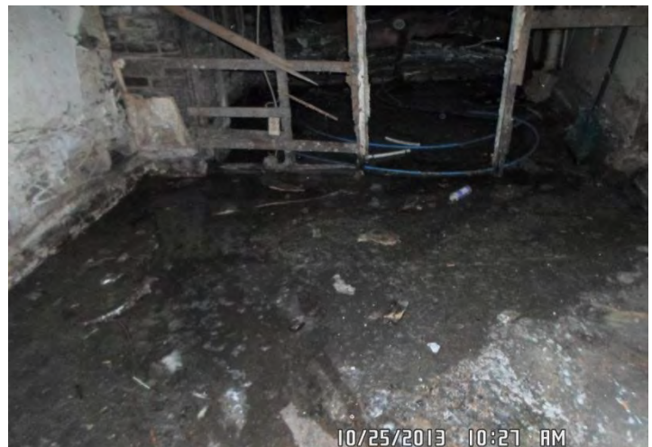
Raw Sewage on a Basement Floor
