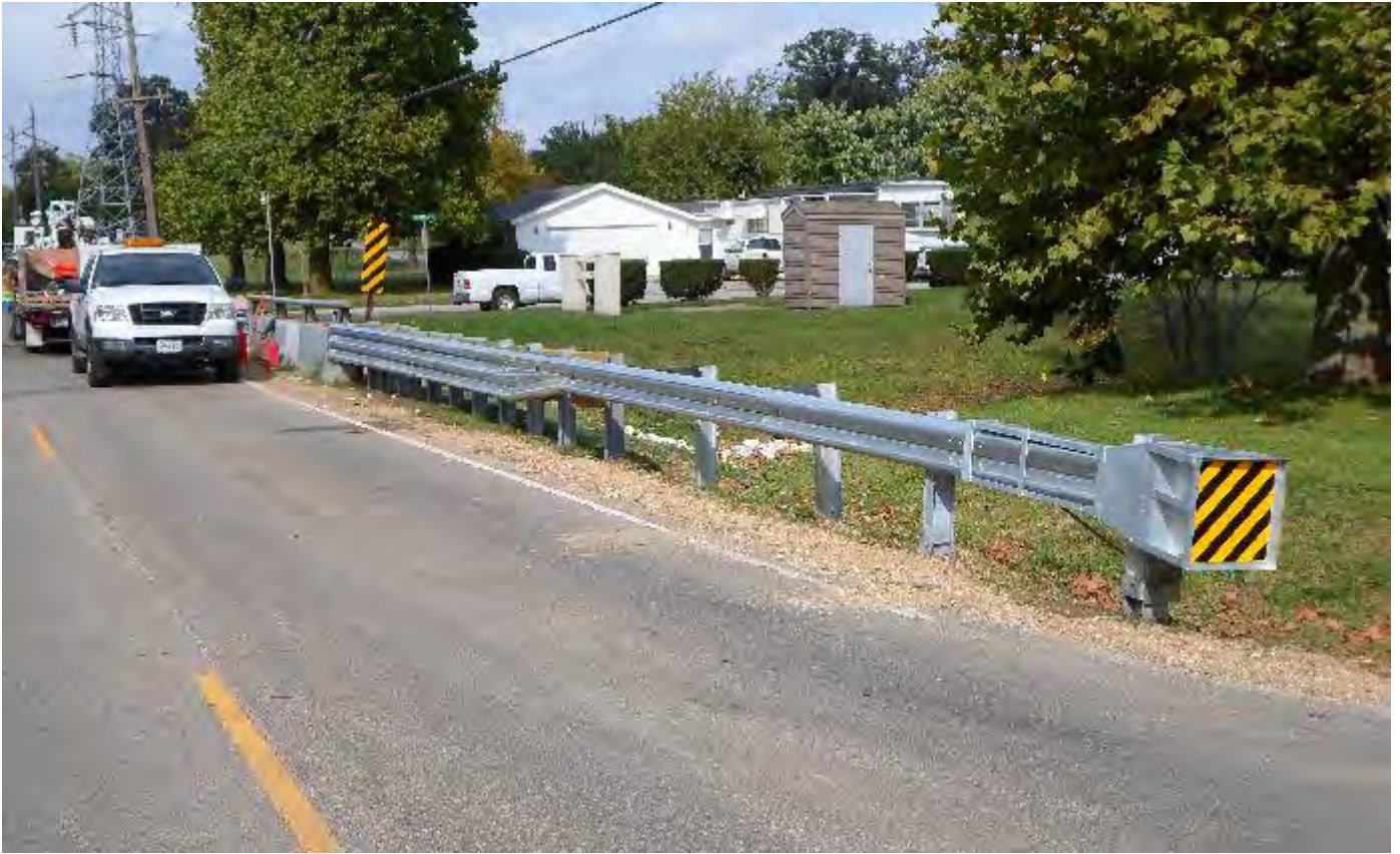
The completed guardrail installed for vehicle safety on Alexander Rd at Goose Creek.
