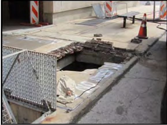
Figure 10: A Collapse Sidewalk Above a Vault
