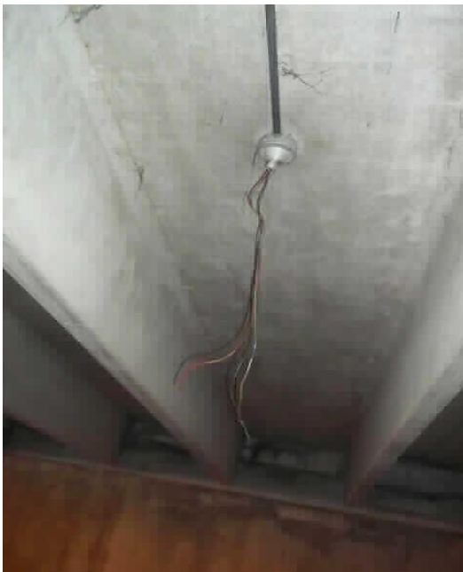
Typical Light Damage at a Parking Garage
