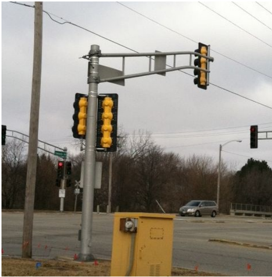
Example of a Traffic Signal
