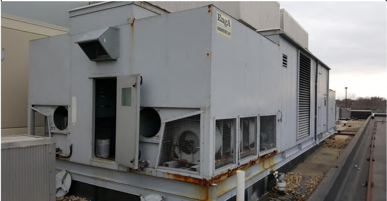
Existing RTU photos
