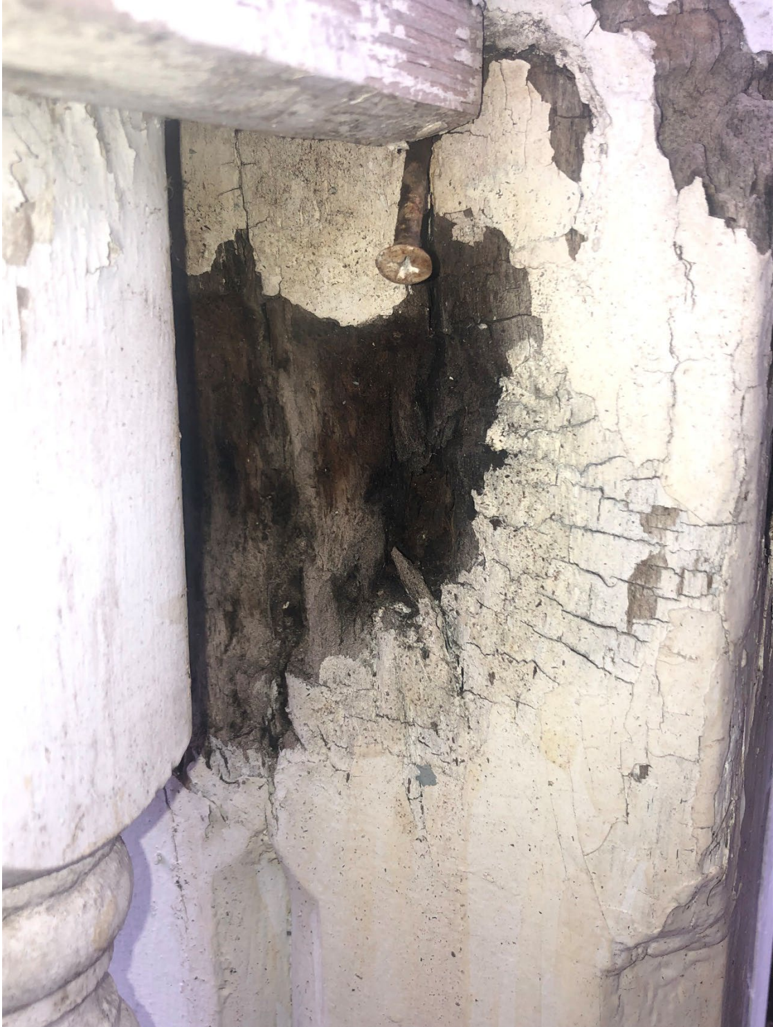
Detail of rot at the midpoint of one column.
