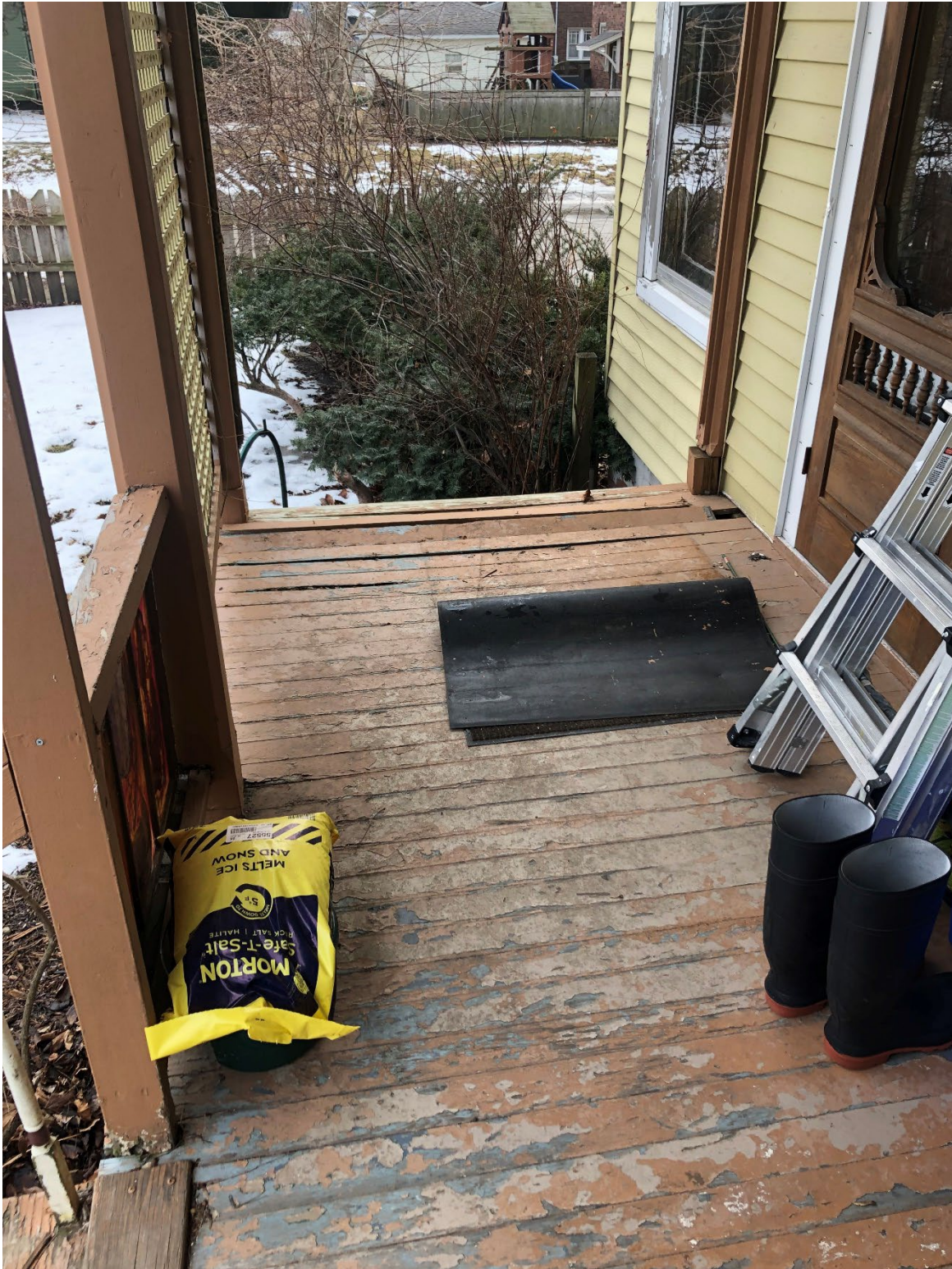
This photo partially shows the three full columns that Brad Williams believes are from an earlier structure. Buckling, wear, and old layers of paint can be seen to the deck boards.
