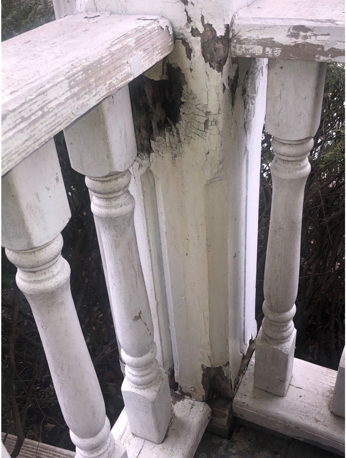
Rot at the base and midpoint of one column.
