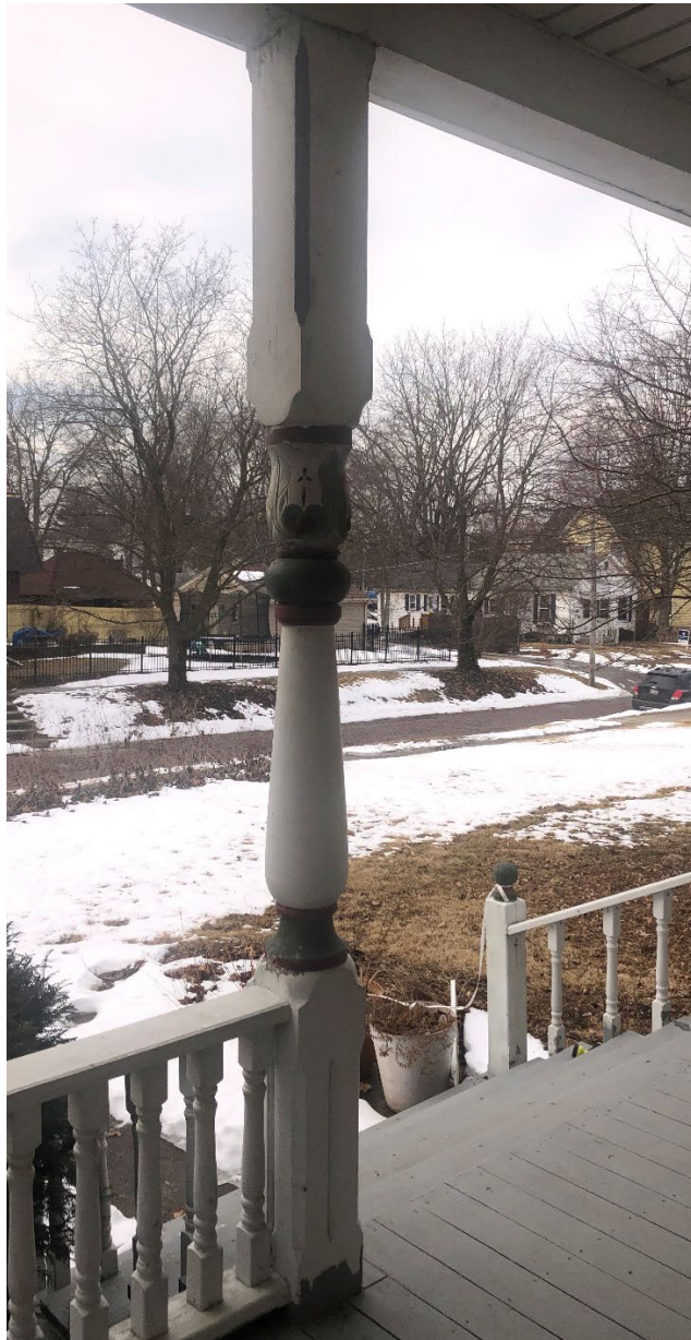
Seven original porch columns remain. Some remain in fairly intact condition, while others exhibit rot to the bases and other wear.
