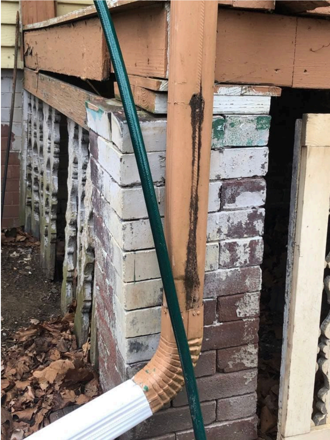
Uneven brick column which will need to be stabilized.
