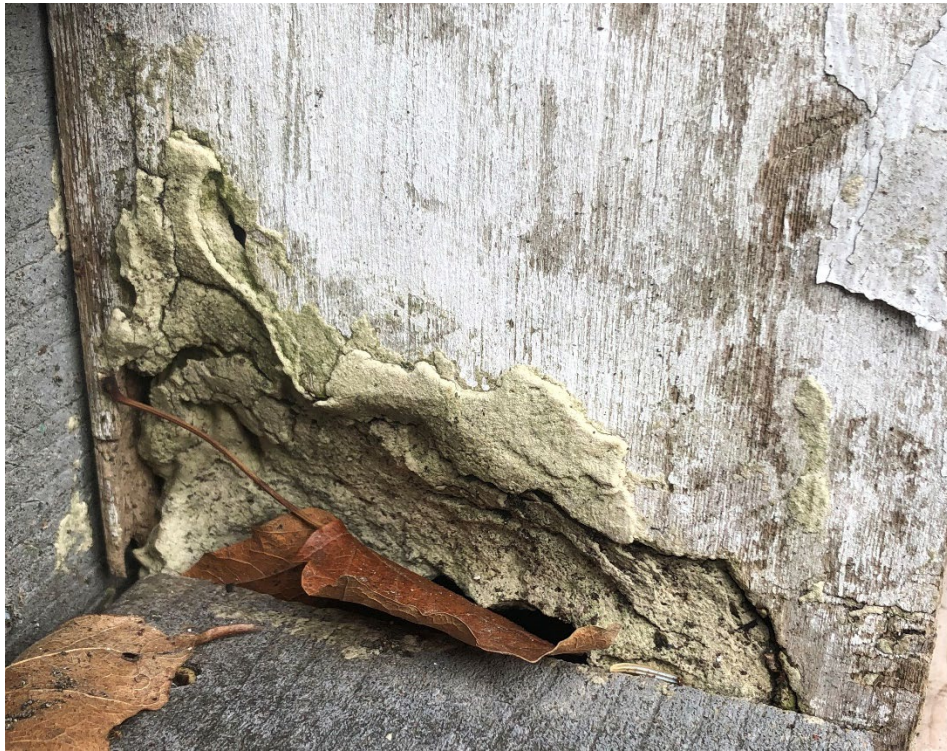
Rot at the base of one of the posts. An unsuccessful attempt at patching can be seen.
