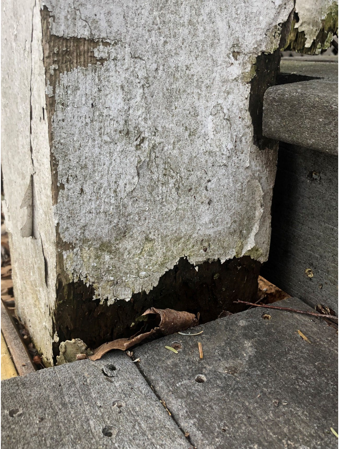
Rot at the base of one of the posts.
