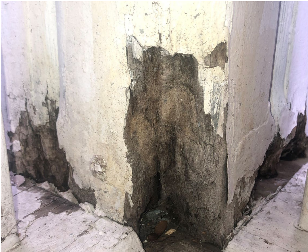
Rot at the base of one of the columns.
