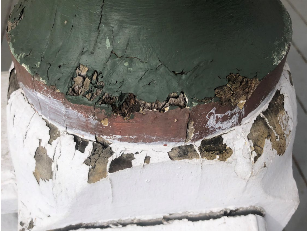
Wear at the midpoint of one of the columns on the south side of the house.
