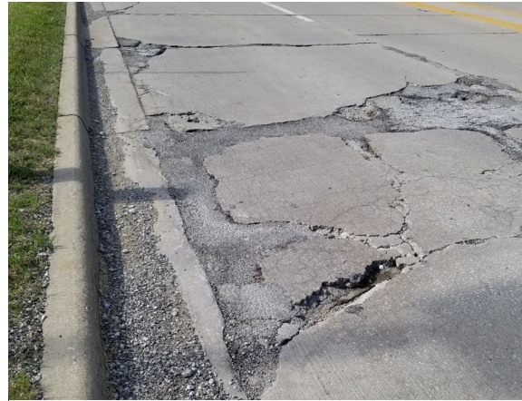
Figure 2: Severe cracking on Wylie Drive north of Maple Hill Road
