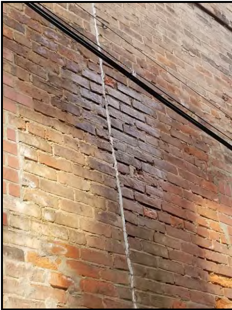
Figure 6 East elevation showing where the water from the downspout drains on to the building.
