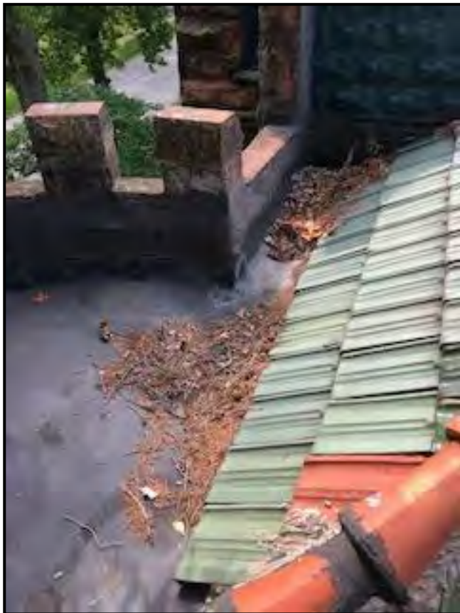
Figure 4 Photo from on top of roof showing the flat portion of the roof and the French ceramic tiles.
