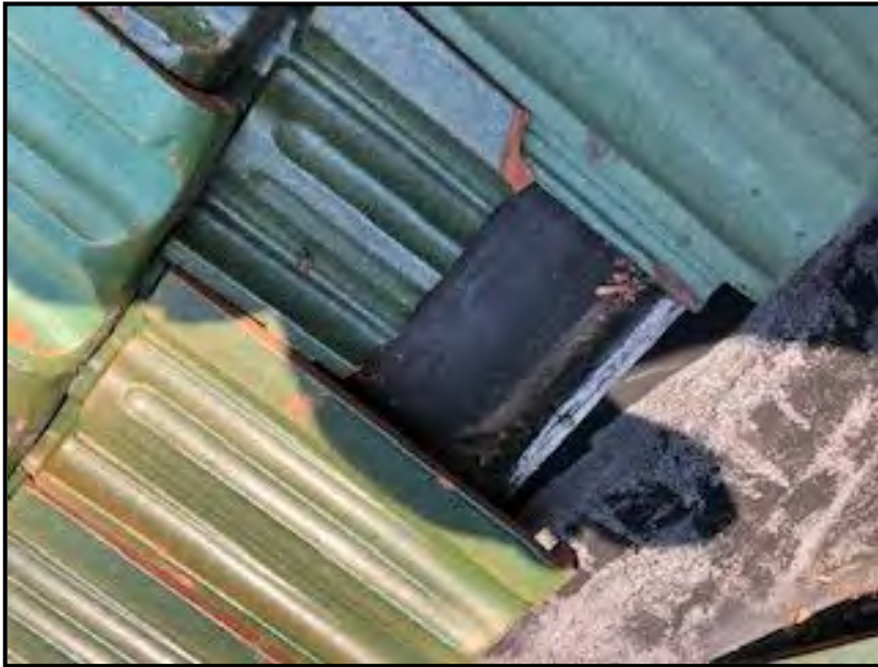
Figure 7 Close up of broken ceramic roof tile.
