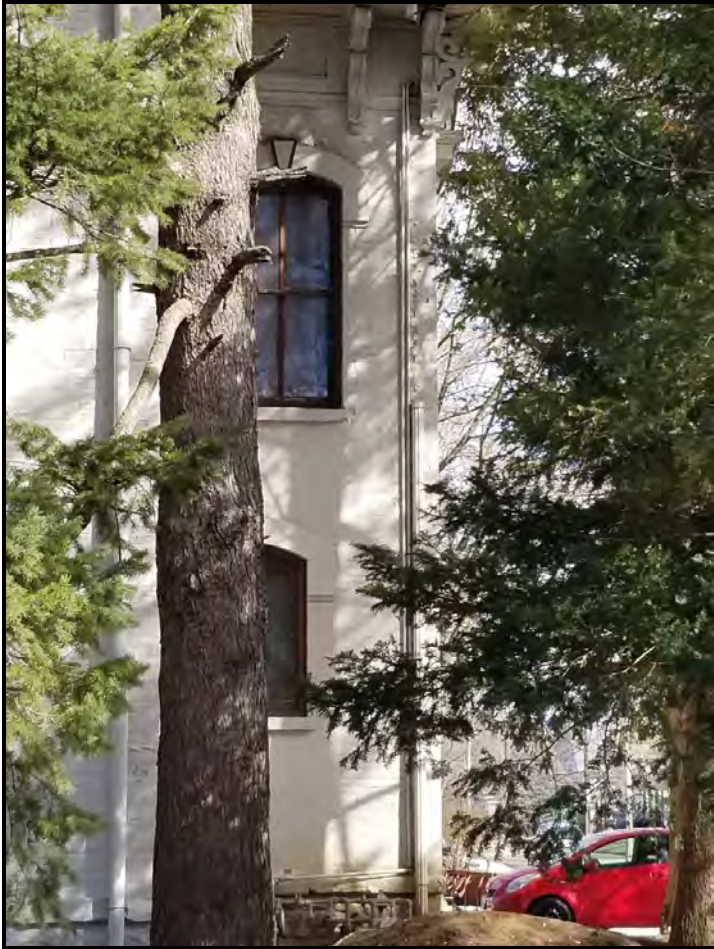
Figure 9 Front facade - portion of downspout missing.
