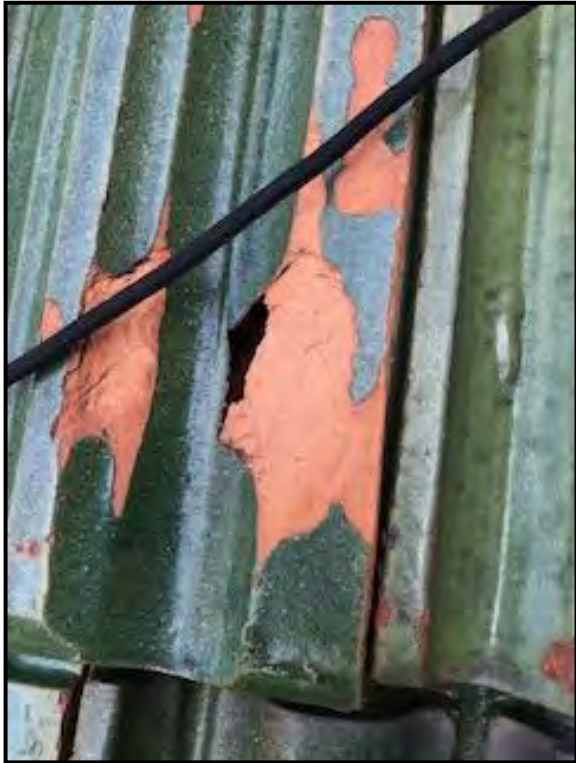
Figure 9 Broken ceramic roof tile.
