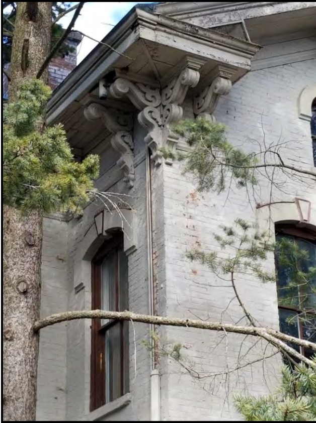
Figure 11 Same section of downspout shown above, showing missing portion.
