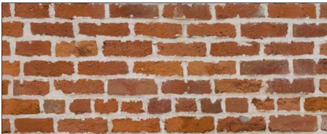
Widened and extended joints – A power tool was used to cut-out the joints during repointing, extending vertical joints. The joints have also been widened and are too large.
