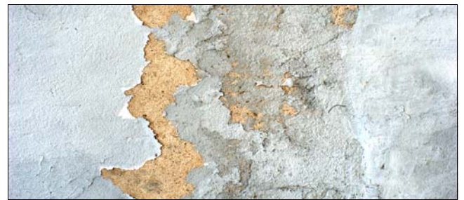
The peeling paint is likely incompatible with the stucco or caused by moisture. Loose and flaking paint should be removed and the cause for failure addressed before repainting.
