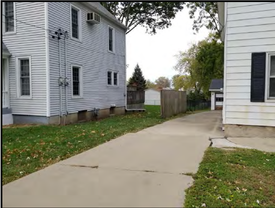
Figure 7 East side of 919 West Wood Street the unfinished side faces the property owner.
