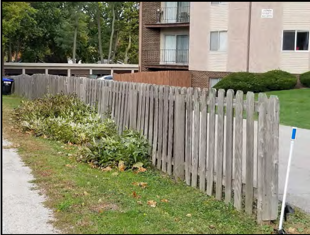
Figure 16 East side of 905 W. Wood Street shadowbox fence finished on both sides.
