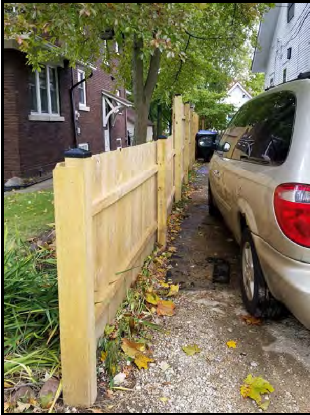
Figure 3 Image showing fence at 916 W. Wood meeting driveway of neighbor at 915 W. Wood.
