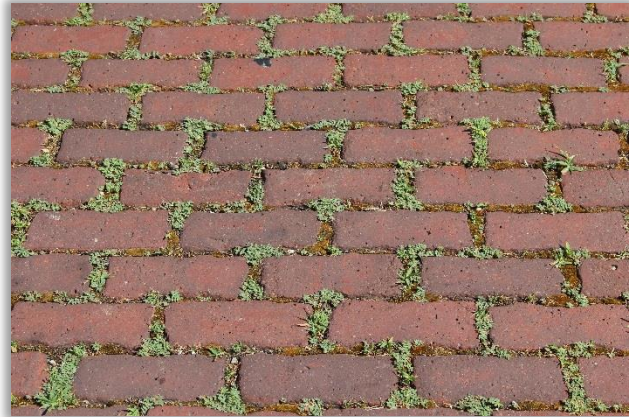
Figure 17: Vegetation between bricks
