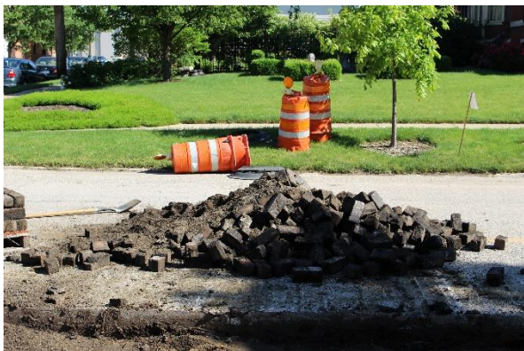
5. Once the bricks are removed, place them in a pile on the nearby road so that they can be palletized.
