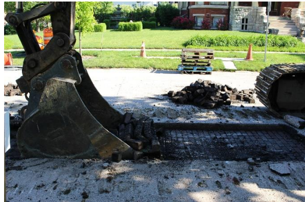
4. The street probably has issues. (There was a reason for the asphalt overlay). Most likely, all of the bricks will have to be removed.
