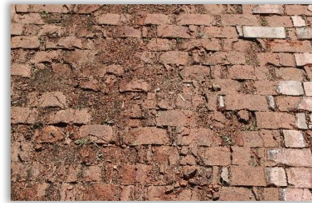
Figure 15: Patio paver bricks after years of use
