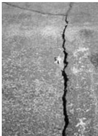
▲ Open crack – 1/2" or more in width.
