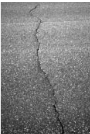
▲ Tight cracks less than 1/4" in width.
