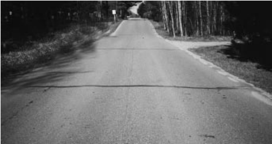
▼ Widely spaced, well-sealed cracks.
