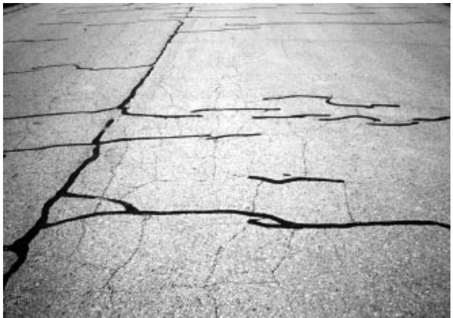
▶ Severe block cracking – 1' or smaller blocks. Tight cracks with no raveling.
