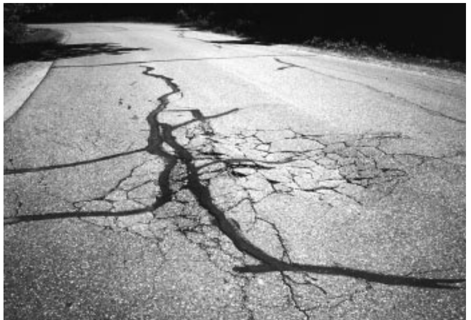
► Frost heave damage from spring break-up.
