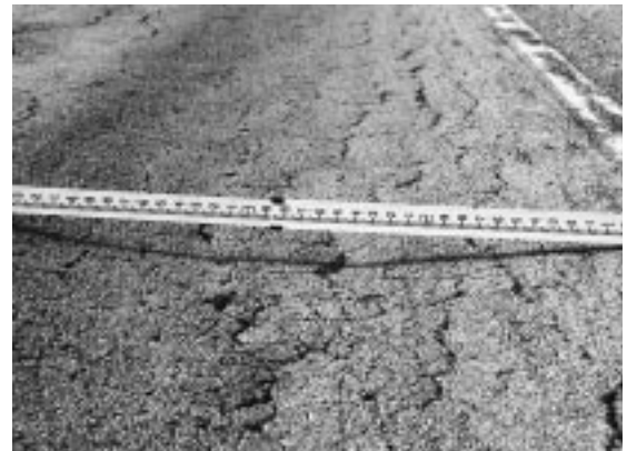
▲ Severe rutting. Strengthen base and reconstruct.
