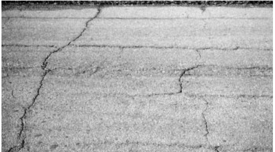
▼ Block cracking with open cracks.
