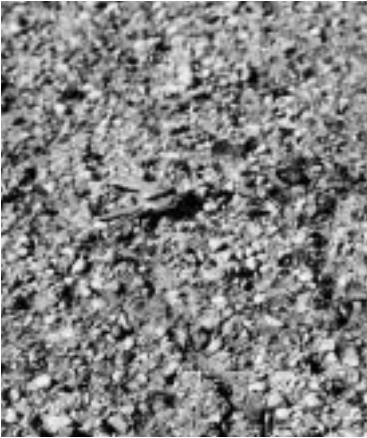
Severe raveling with ▼ extreme loss of aggregate.
