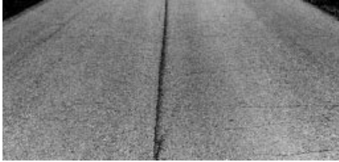
Centerline crack (still tight). ▶
