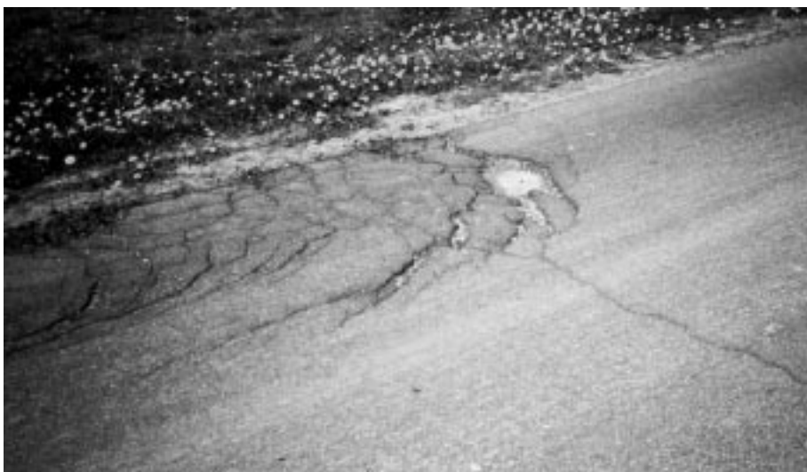
► Crescent-shaped cracks characteristic of slippage.
