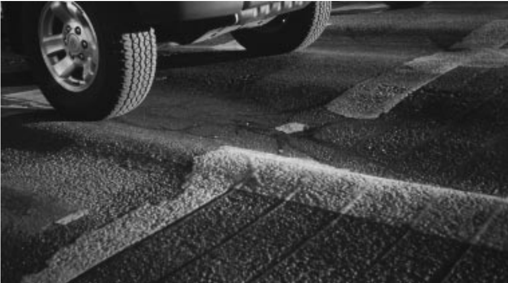
◀ Severe rutting over 2" caused by poor mix design.
