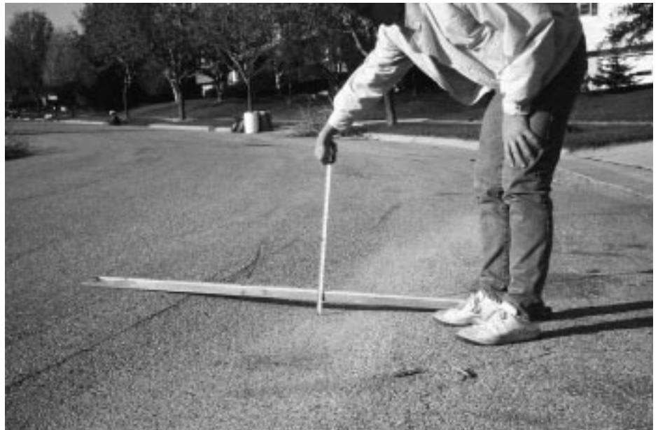
► Severe settling from utility trench.
