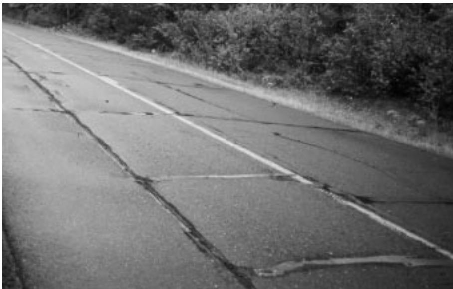
► Concrete joints reflected through bituminous overlay.
