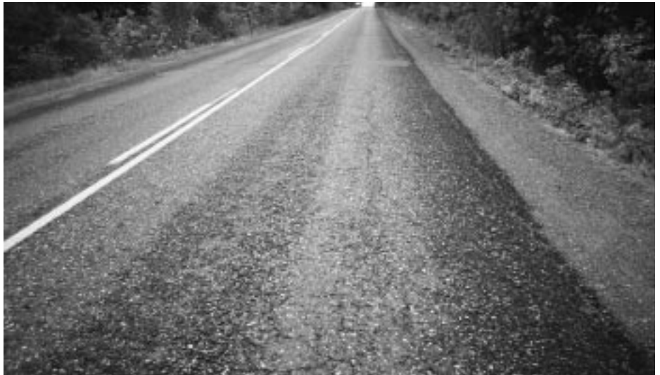
► Moderate to severe raveling in wheel paths.
