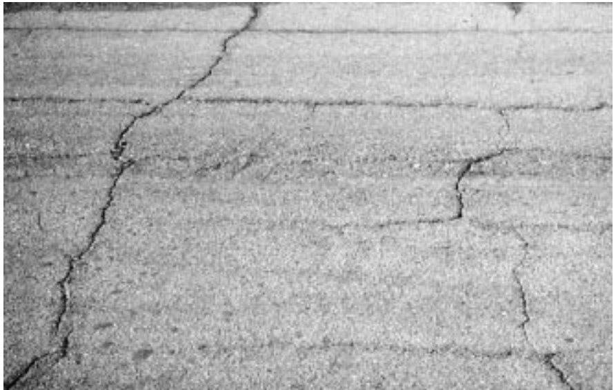
▶ Intermediate-size block cracking, 1'-5' across with open cracks.
