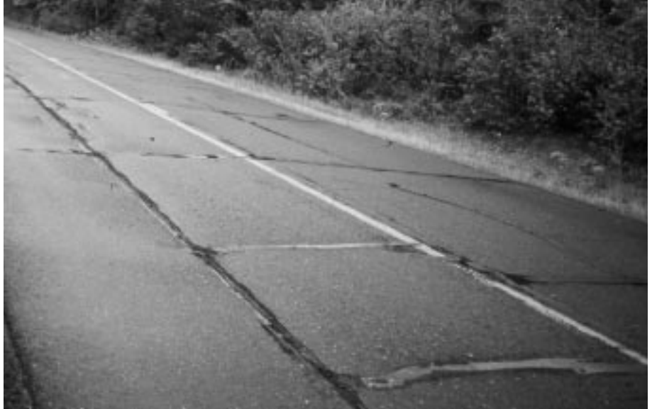
► Concrete joints reflected through bituminous overlay.
