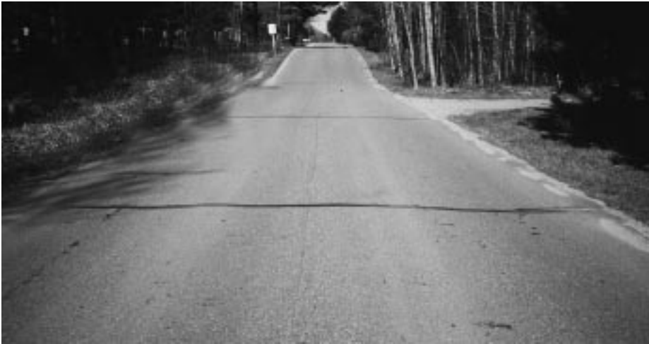
▼ Widely spaced, well-sealed cracks.
