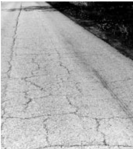
▲ Extensive block cracking in an irregular pattern.
