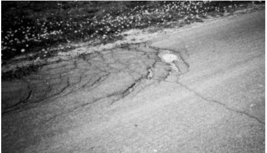
► Crescent-shaped cracks characteristic of slippage.
