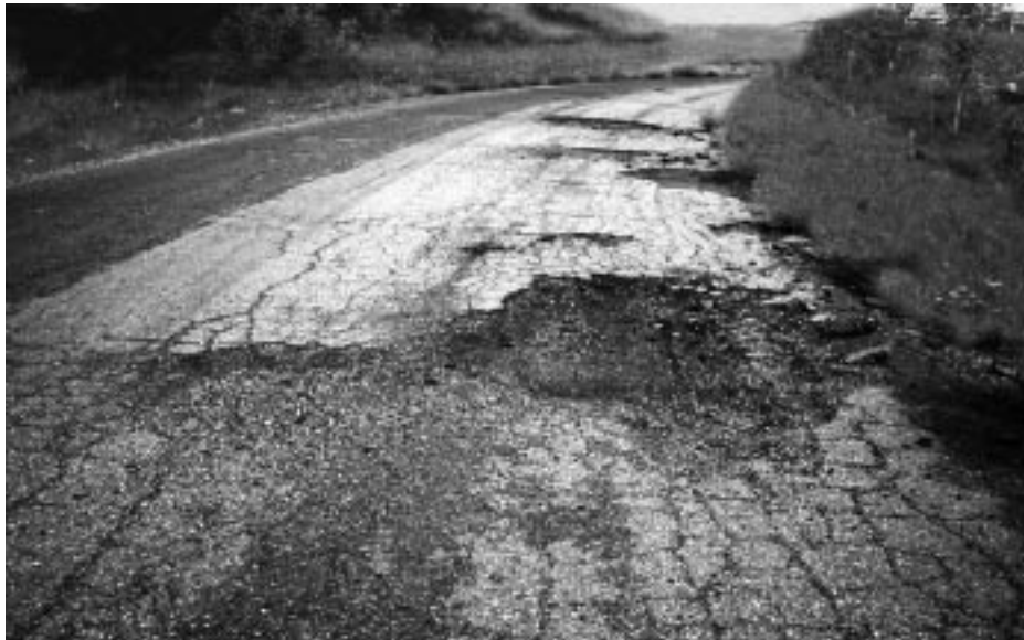
◀ Large, isolated pothole, extends through base. Note adjacent alligator cracks which commonly deteriorate into potholes.
