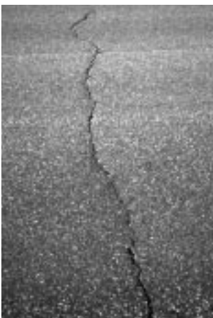
▲ Tight cracks less than 1/4" in width.
