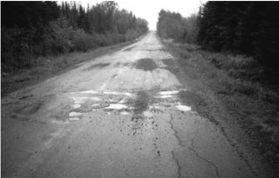
◀ Multiple potholes show pavement failure, probably due to poor subgrade soils, frost heave, and bad drainage.
