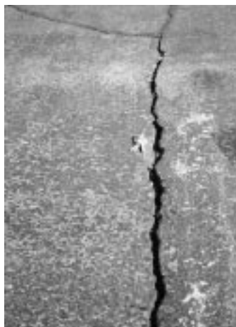
▲ Open crack – 1/2" or more in width.
