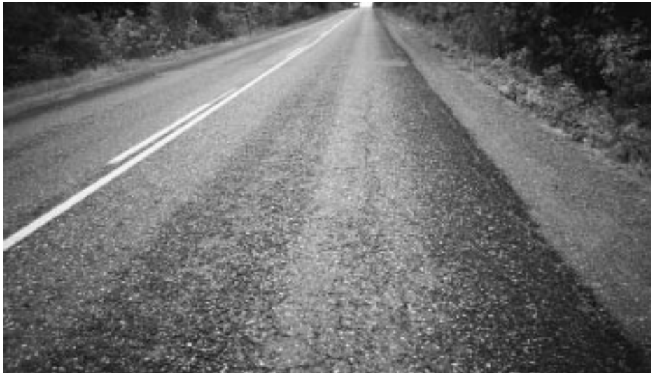
► Moderate to severe raveling in wheel paths.
