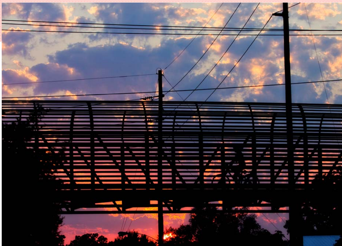
Bridge over Oakland Ave for Constitution Trail, photo courtesy of: Jeff Buydos, September 2011
