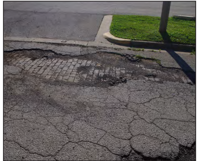
The asphalt pavement on North East Street, located on the 804 North East Street property, has disintegrated exposing the old brick street surface.
