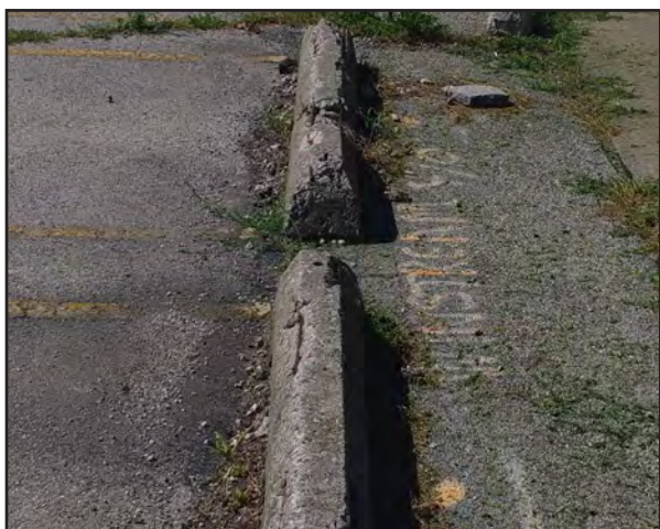
Left: The curb stops for 103 West Chestnut Street are deteriorated, exposing their steel reinforcing bars.
