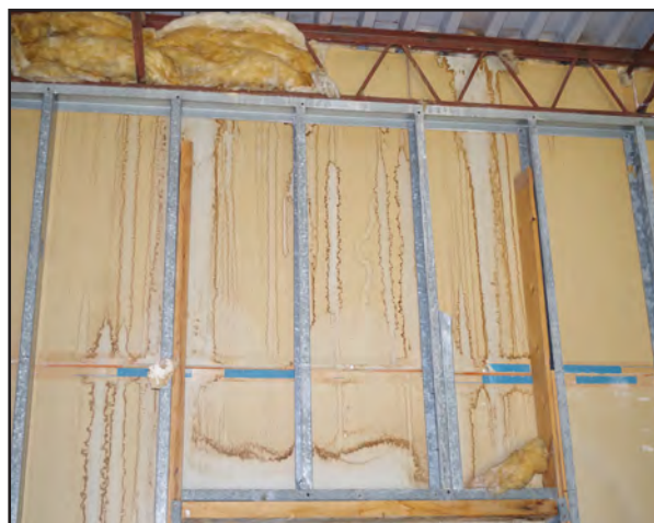
Right: Water stained drywall, due to a roof leak, in the Creativity Center.
