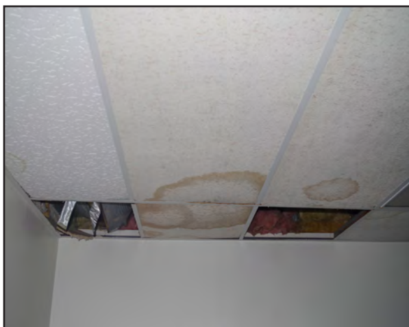
Left: Water damaged and collapsed ceiling tiles at the Creativity Center.
