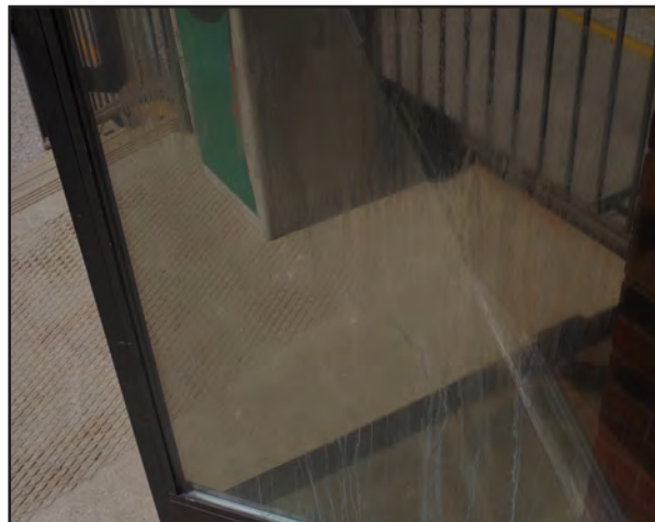
Right: Moisture inside of the glass door of the Creativity Center, indicating the seals have failed.
