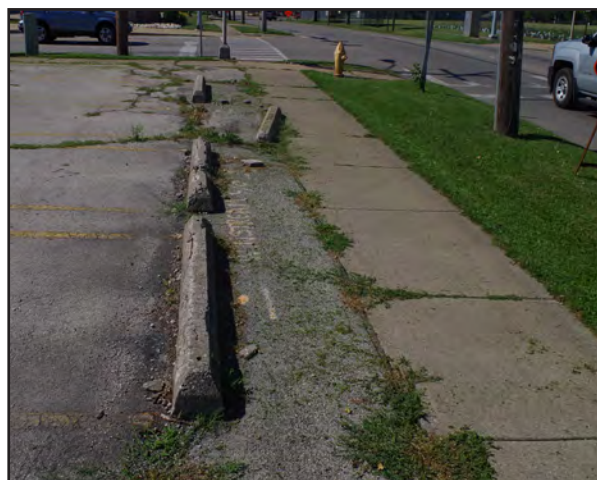
Right: A dislodged curb stop located at 103 West Chestnut Street.
