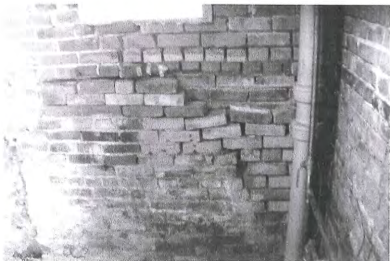
BROKEN & REMOVED BRICK
