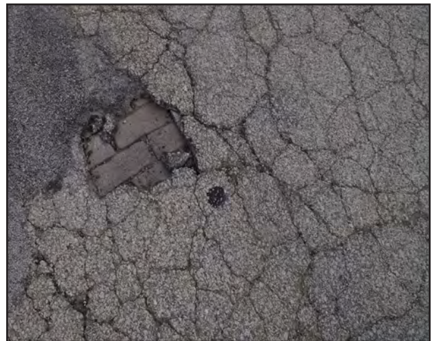
Right: Deteriorated street pavement along East Jefferson Street.
