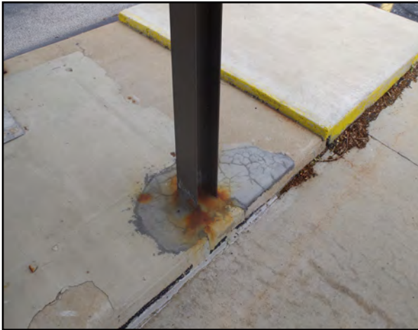
Left: The columns supporting the drive through canopy are rusted at the base.
