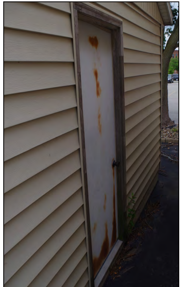
Right: The exterior door, on the garage for the vacant bank, has rusted.
