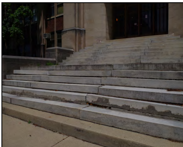
Left: The front entry steps to the former school are deteriorated and not level.
