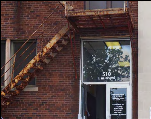
Left: A rear fire escape that has rusted and become deteriorated.
