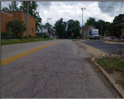
Above: The pavement along North McLean Street is deteriorated.
