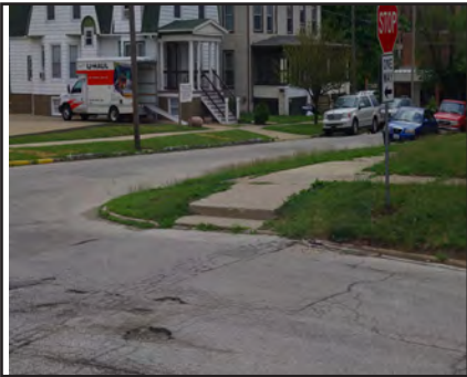
Below: The pavement and curbs are deteriorated at the intersection of Gridley and Jefferson.
