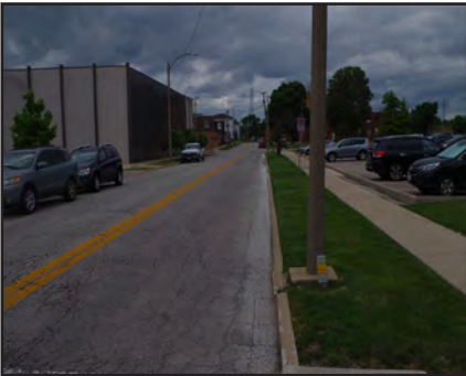
Below: The pavement along North Gridley Street is deteriorated.
