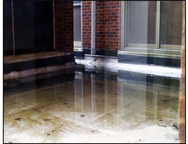
Right: Standing water on the roof of the school building.
