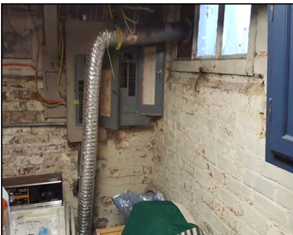
Left: Flexible exhaust venting ran to the window of the salon presents a carbon monoxide hazard.
