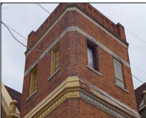
Left: A missing window in the church tower allows the weather and wildlife to enter into the structure.
