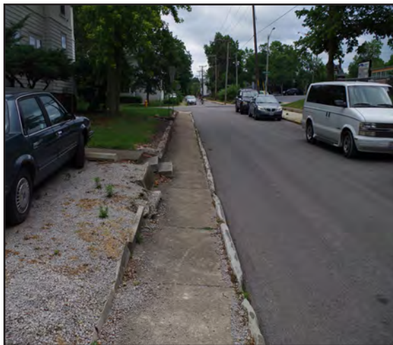
Left: Deteriorated curbs along North McLean Street.
