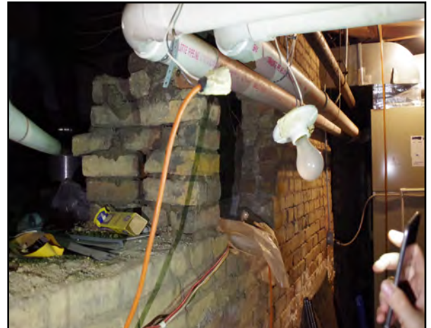
Right: A basement light improperly wired into an extension cord.
