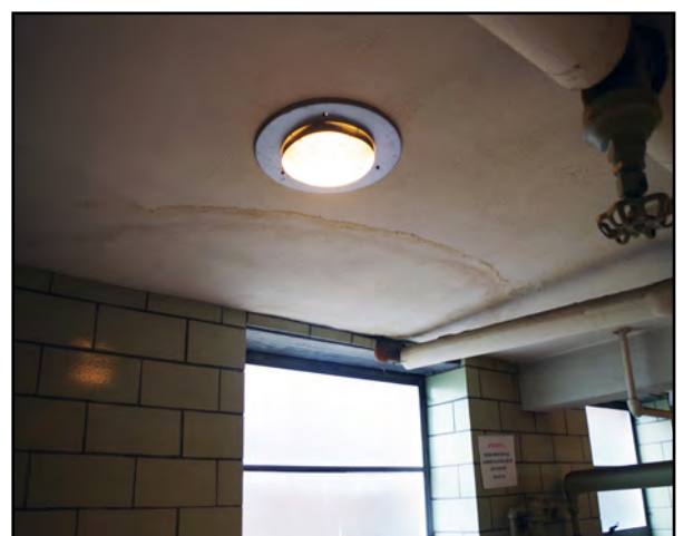
Right: Water damage to the ceiling in the church's basement kitchen.
