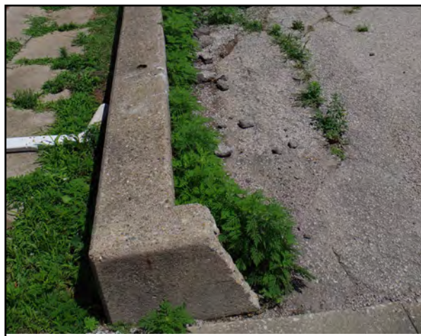
Left: The retaining wall on the north side of 500 East Jefferson is leaning.
