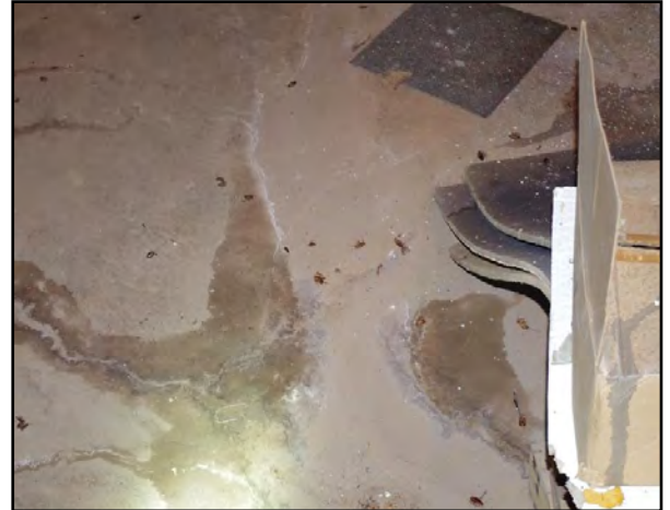
Right: The basement of the former school contains hundreds of dead cockroaches.
