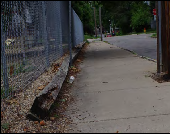
Left: Rotted rail-road ties along the school fence.
