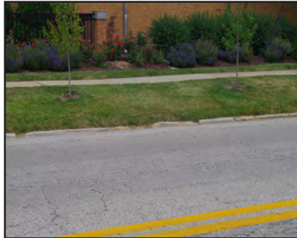
Above: The curbs along North McLean Street are deteriorated.
