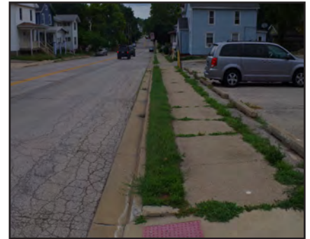
Below: Deteriorated pavement along North McLean Street.
