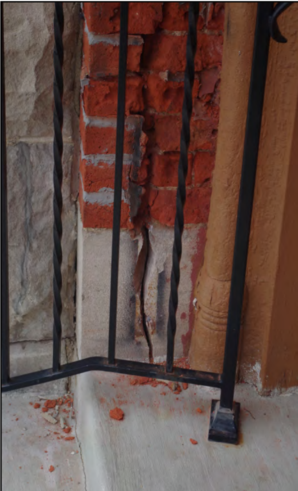
Left: Disintegrating exterior brick wall of the church.
