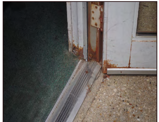
Right: A rusted door frame located at a church entrance.
