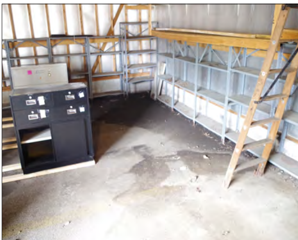
Left: Due to improper grading, water is running into the storage garage for the vacant bank.
