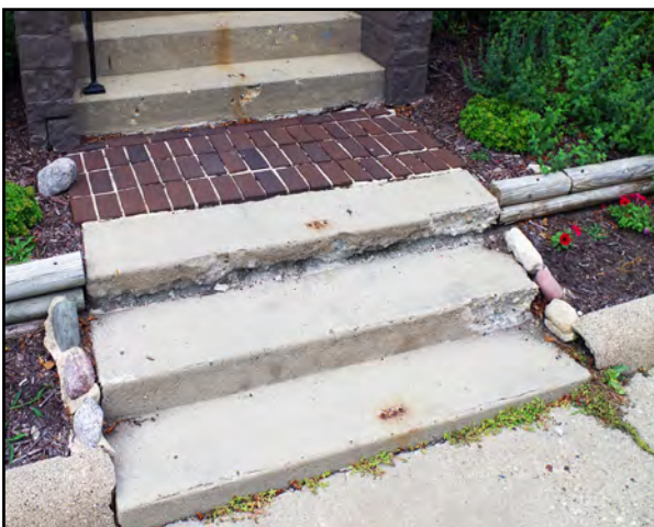
Left: The steps, leading to the entrance, are deteriorated.
