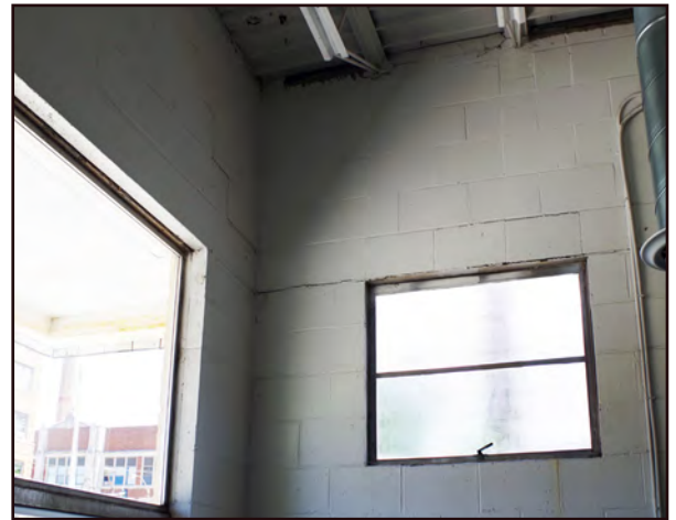
Right: Step cracking in the interior CMU walls.
