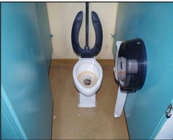
Left: A dry toilet allowing sewer gasses into the building.
