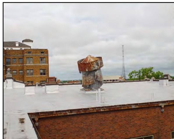
Right: The exhaust hood on the top of the former school is leaning.
