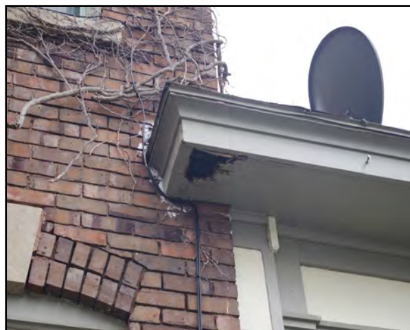
Right: Portions of the enclosed soffit and fascia are rotted out.
