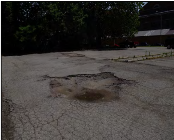
Left: The parking lot at 500 East Jefferson is deteriorated and contains large potholes.
