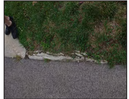
Above: The curbs along East Front Street are deteriorated.
