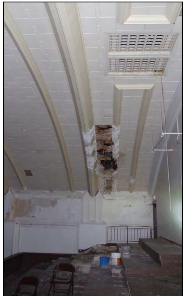
Right: Damage to the balcony ceiling, in the auditorium, of the former school.
