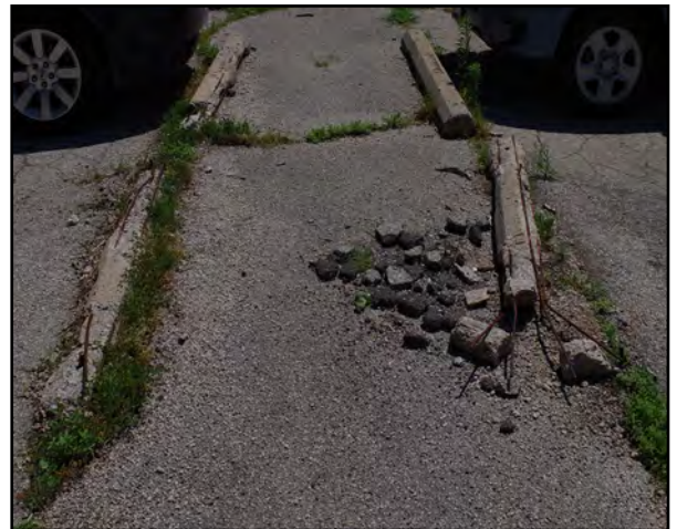
Right: The parking stops at 500 East Jefferson are crumbling and deteriorated.
