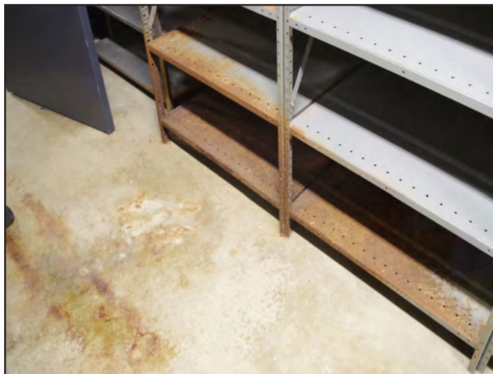
The metal shelving in the basement has rusted as a result of the moisture infiltration.
