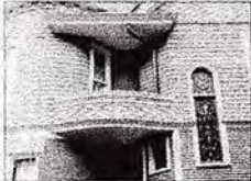
Restoring details like this balcony in the Oscar Mardel home is expensive but worth the effort for those who appreciate the history of the structures.
