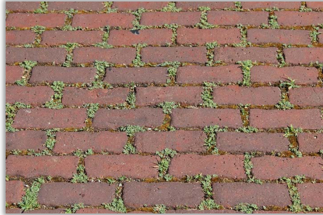
Figure 17: Vegetation between bricks
