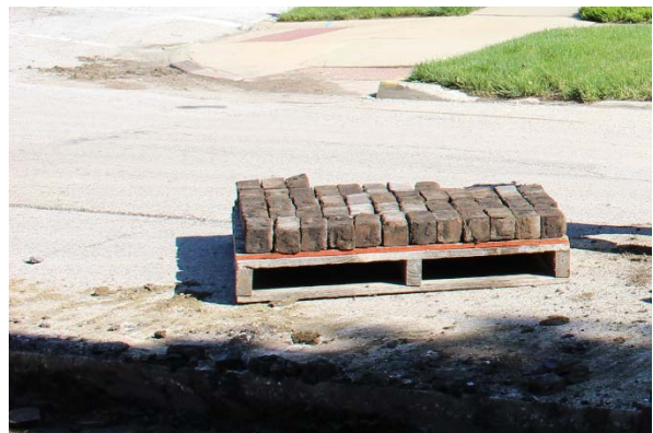
6. Carefully stack undamaged bricks on a pallet. Count on having to discard 30 percent of the bricks because of various types of damage.
