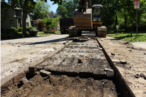
1. This process requires a backhoe with teeth in good condition or other, similar equipment.
