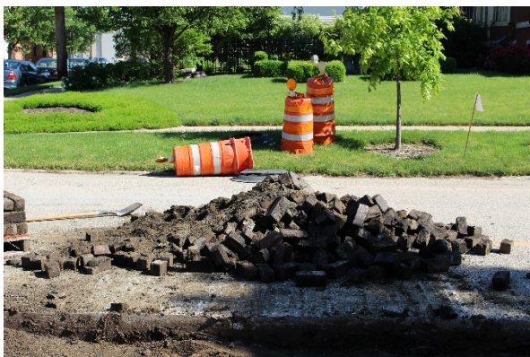
5. Once the bricks are removed, place them in a pile on the nearby road so that they can be palletized. Alternatively, haul them away to another location to be palletized later.
