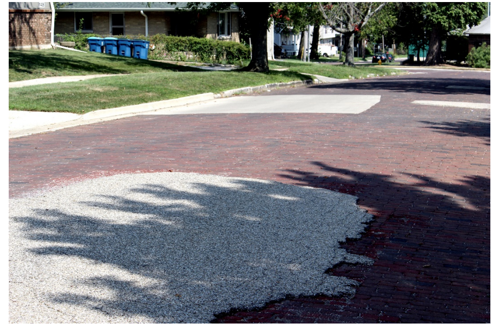
Asphalt and concrete patches
