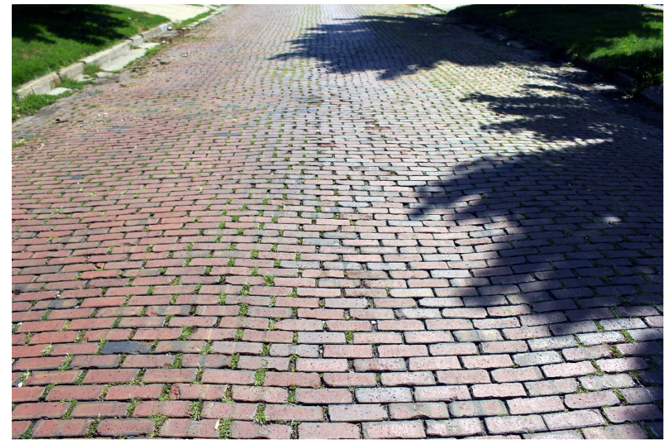
Rutting and unevenness
