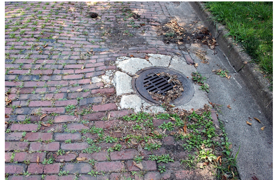
Storm drain unevenness
