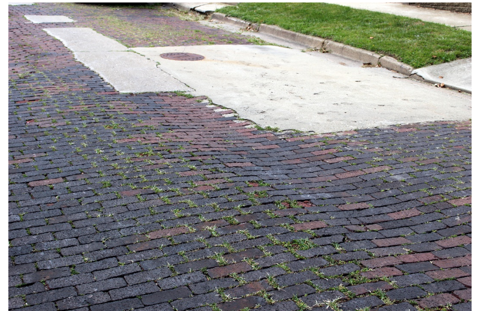
Concrete patches and very minor rutting 9
