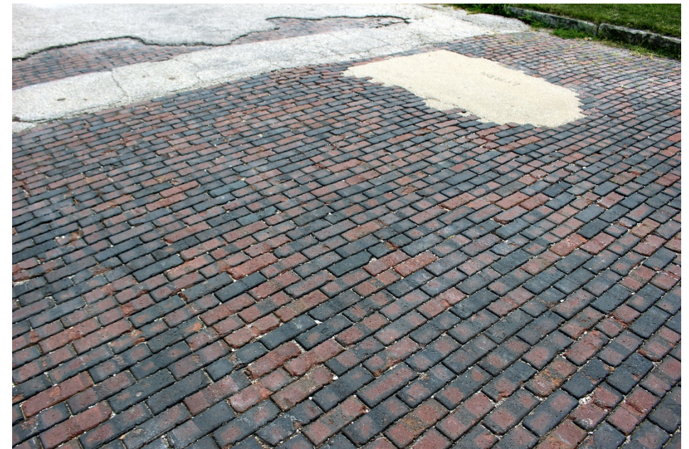
Concrete and asphalt patches
