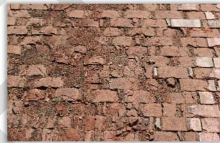
Figure 21: Patio paver bricks after years of use
