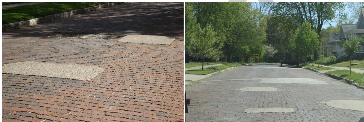
Figure 11: Condition of Monroe St., from Clinton St. to Robinson St. in Spring 2017
