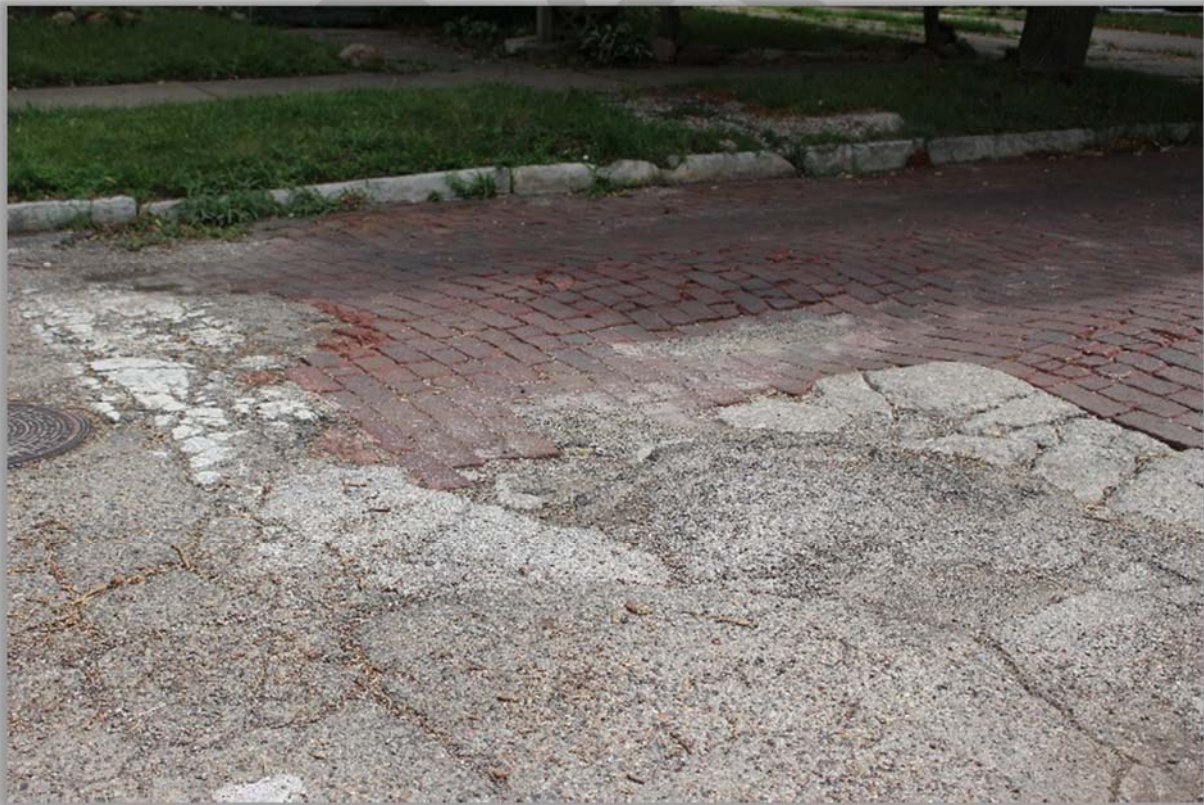
Figure 22: Rutting near stop sign on Monroe St. at Clinton St.
