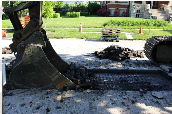
4. The street probably has issues. (There was a reason for the asphalt overlay). Most likely, all of the bricks will have to be removed.
