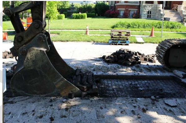
4. The street probably has issues. (There was a reason for the asphalt overlay). Most likely, all of the bricks will have to be removed.
