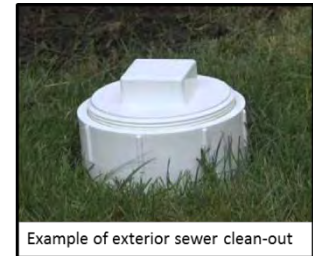
Example of exterior sewer clean-out
