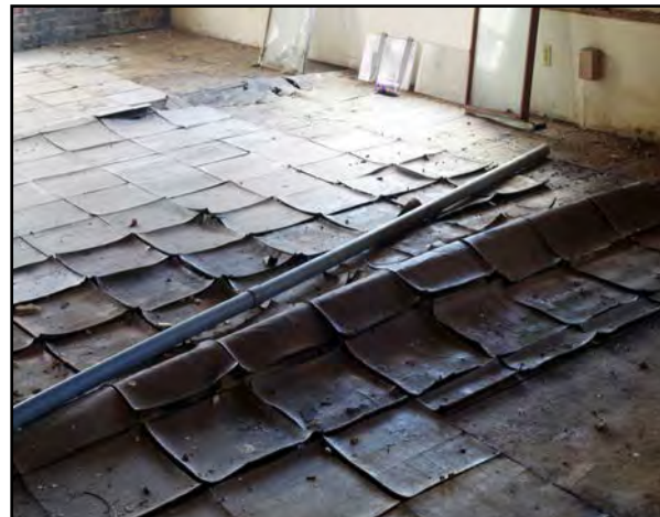
Right: Warped and water damaged tiles on the second story of the Front N Center Building. Note: underlying wood floor is buckling.
