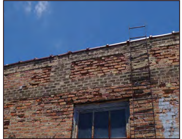
Right: The bricks and mortar on the upper level of the Front N Center Building are deteriorated.
