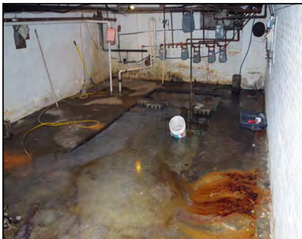
Left: Standing water in the basement of the Golden Rule Building.
