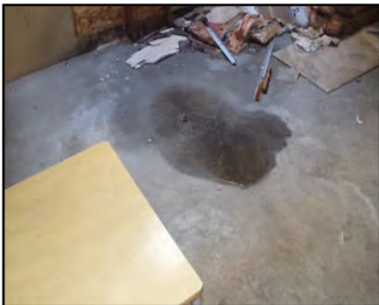
Below: Water on the floor of the former Elks lodge due to roof leaks.
