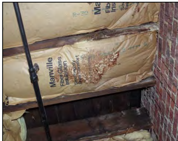
Right: Water damage to the ceiling in the attic of the Golden Rule Building.
