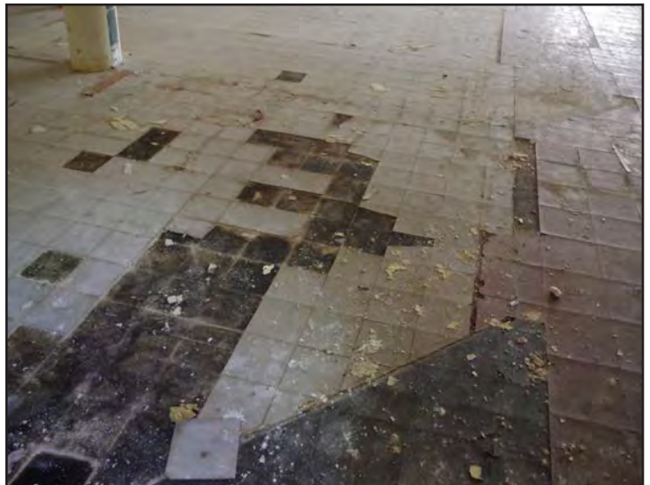
Floor tiles have become dislodged inside of the Front N Center Building. The flooring is suspect for containing asbestos. (1st Floor)
