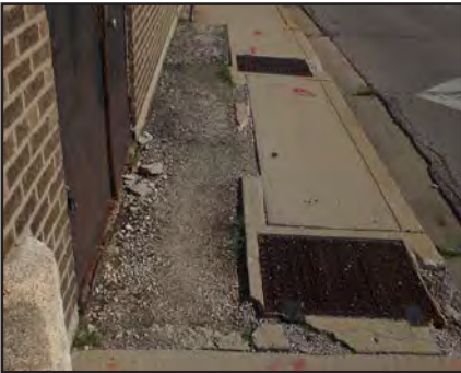
Below: The sidewalk along Front St., between Madison and Center, is deteriorated.
