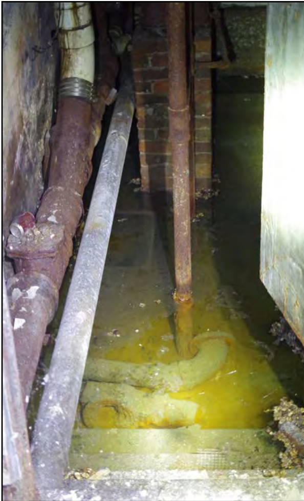
Left: Standing water in the lower level of the Front N Center building.
