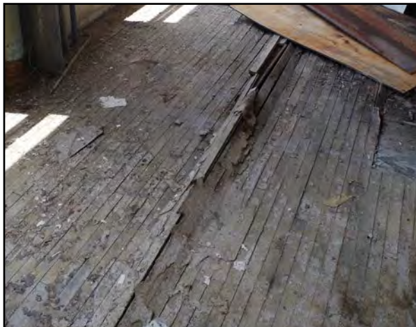
Left: The wood floor on the second story of the Front N Center Building is buckling.
