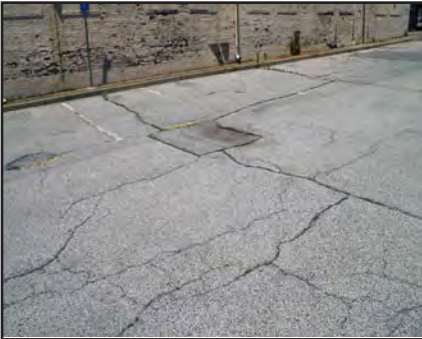
Above: The parking lot at 301 W. Front has deteriorated pavement.
