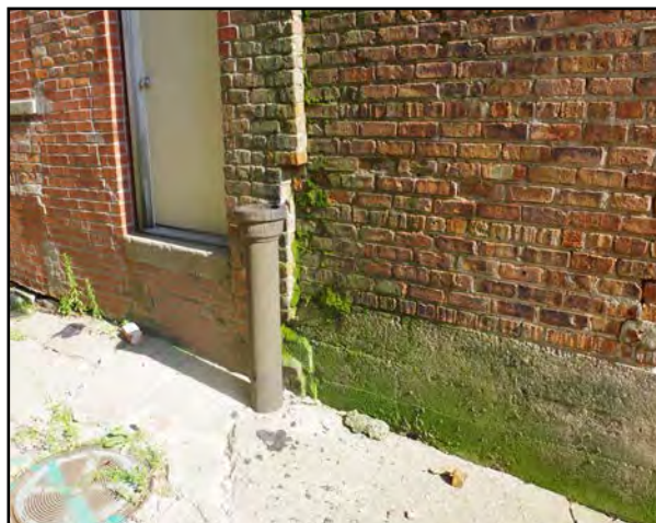
Left: Moss growing on the side of 110 N. Center next to a missing downspout.
