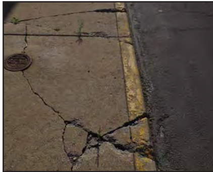
Below: The sidewalk and curbing along N. Roosevelt are deteriorated.
