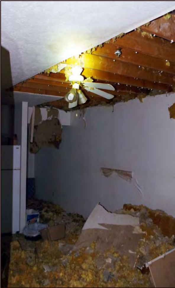
Left: Water damage to the upper floor apartments on the Front N Center Building.
