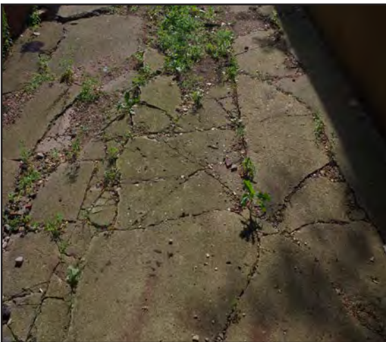
Left: A deteriorated alley between N. Center St and N. Madison St.
