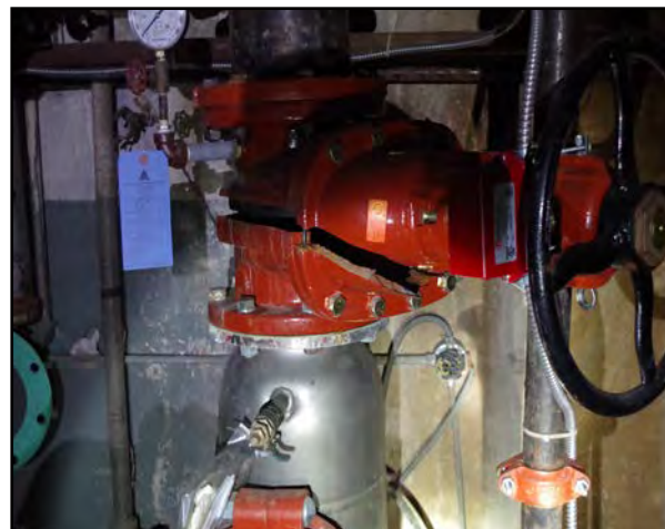
Right: The water main supply in the Front N Center Building is severely damaged and inoperable. (Lower Level)
