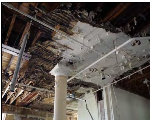
Left: The plaster ceiling on the second floor of the Front N Center Building has almost completely collapsed.
