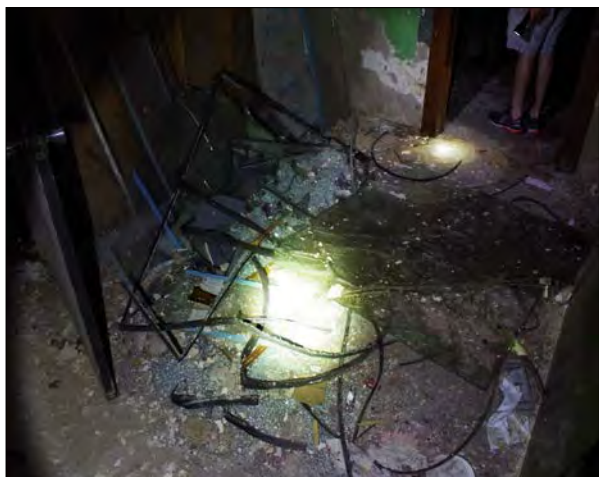
Left: Broken glass on the floor of the Front N Center Building. (Lower Level)
