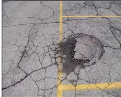
Above: The parking lot in the rear of 402 W. Washington is deteriorated.
