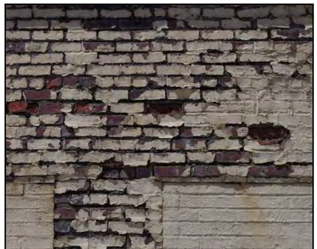
Right: The exterior coating and bricks on the former Elks Lodge are deteriorated.
