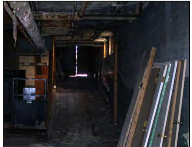
Right: Rear loading doors accessing the lower level of Front N Center do not seal the building from the weather or rodents.
