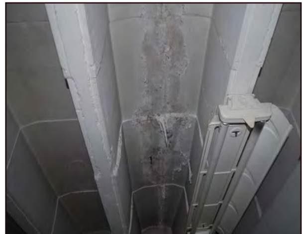
Right: Water penetrating the basement ceiling of the Commerce Bank Building has resulted in the formation of mineral stalactites.
