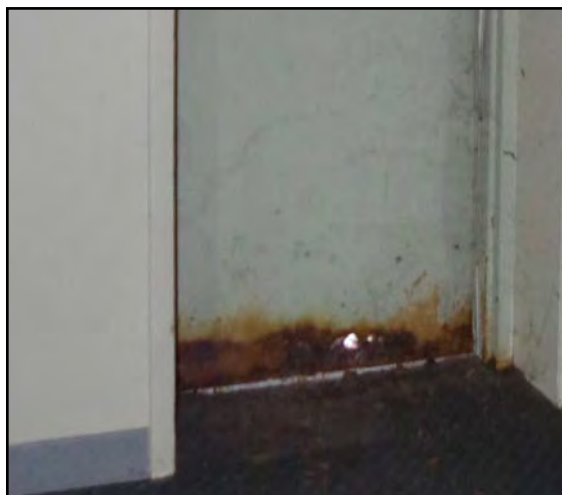
Left: The front door on the former Elks Lodge is rusted exposing exterior elements and allowing access for rodents.
