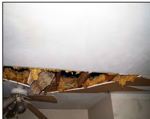
Right: Water damage to the upper floor apartments on the Front N Center Building.
