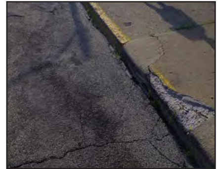
Below: Deteriorated pavement and curbing along N. Center Street.
