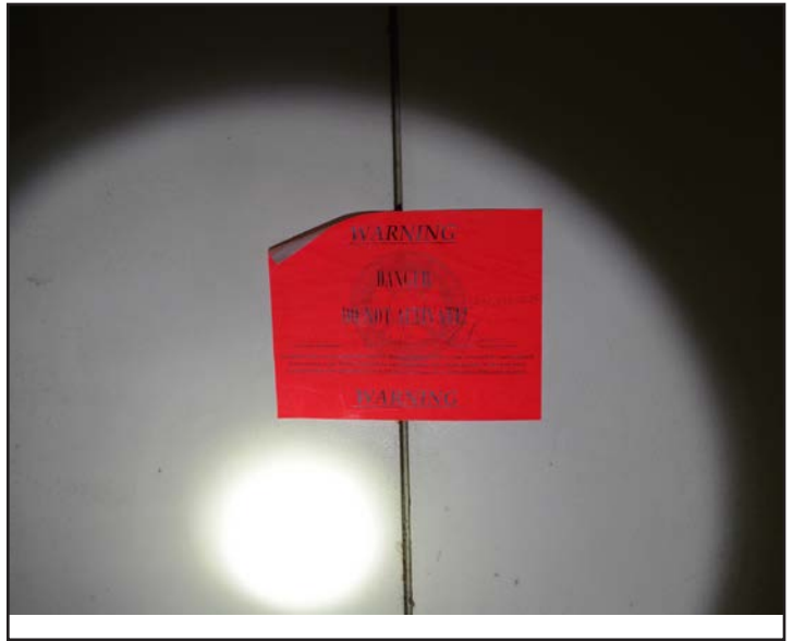
The elevators in the Front N Center Building have been removed from service.
