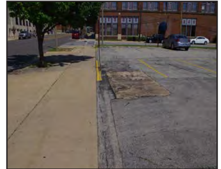
Above: The paving in the parking lots covers the entire parcel, not meeting landscaping requirements.
