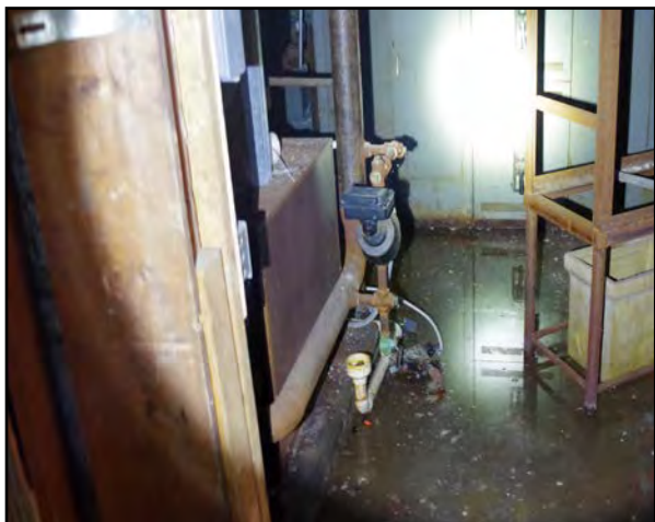
Left: Standing water in the room containing the main electrical service. (Lower Level)
