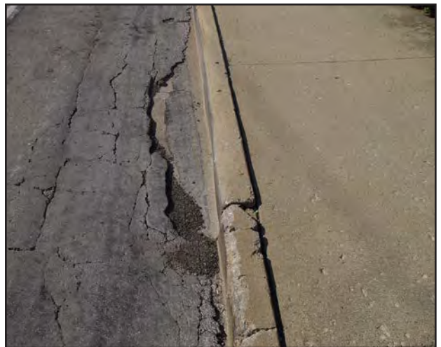
Right: The edge of the pavement along N. Roosevelt is deteriorated.
