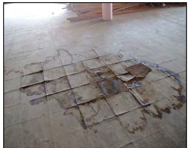
Right: Water damaged floor tiles that have become loose. (2nd Floor)
